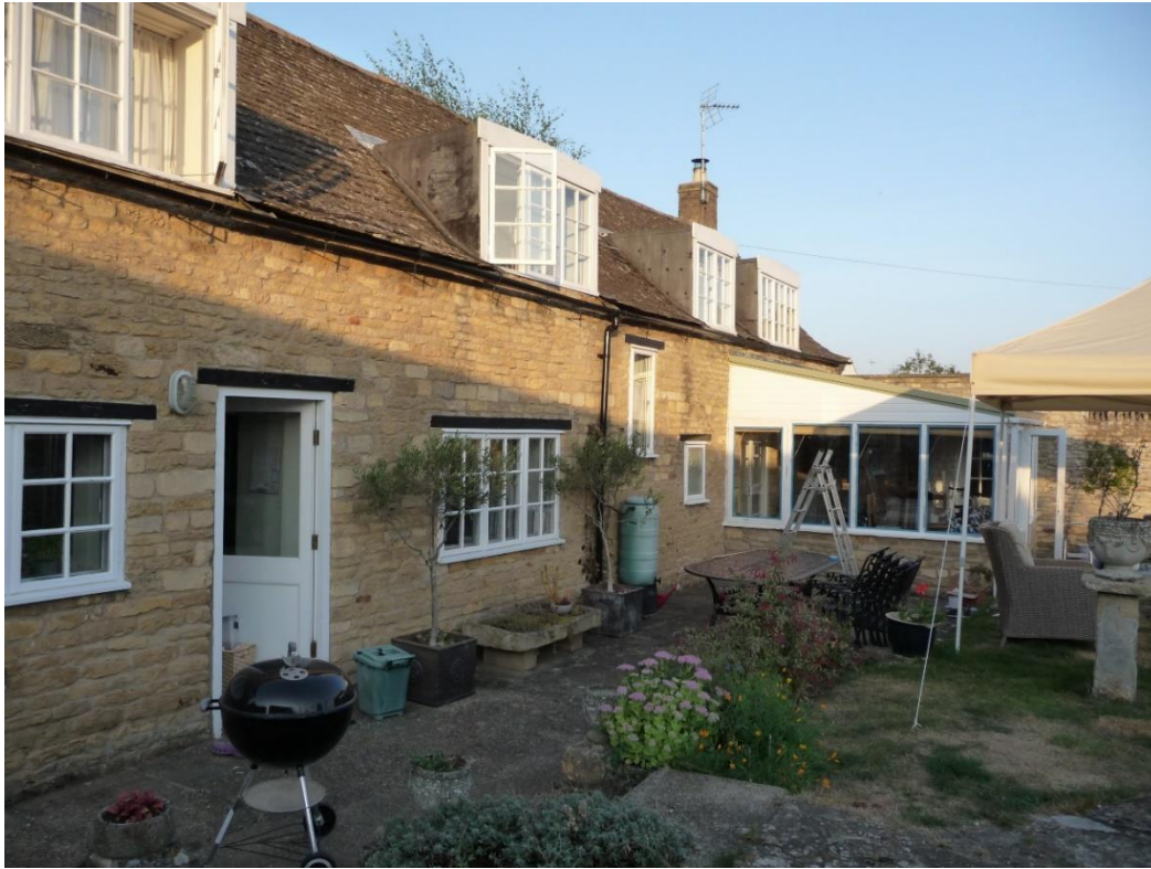
Figure 4. A slightly angled view of the same. The lintels are very uniform, and presumably date from the 1970s refenestration.
