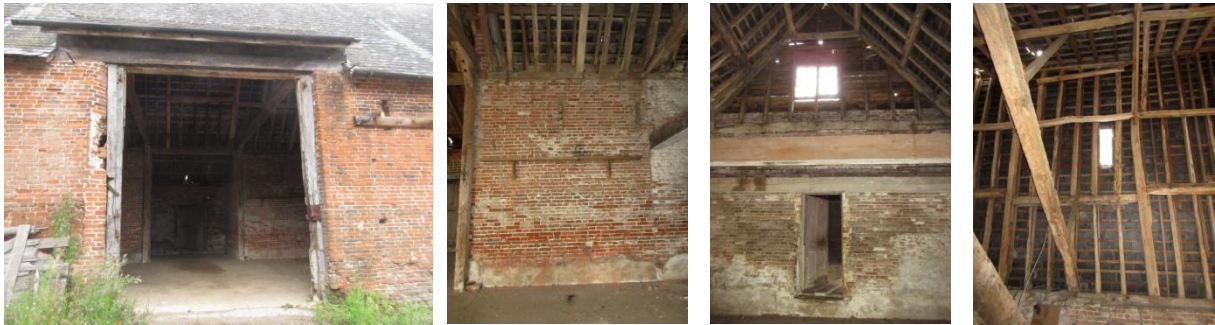
Left to Right: main entrance to barn with doors missing; looking towards N wall in bay 5 where it is proposed to insert a door into the living room of Unit 2 at ground floor level; looking E showing doorway into shed G (to be demolished); section of original roof structure to E of entrance bay showing clasped purlin with lower tier of staggered butt purlins
