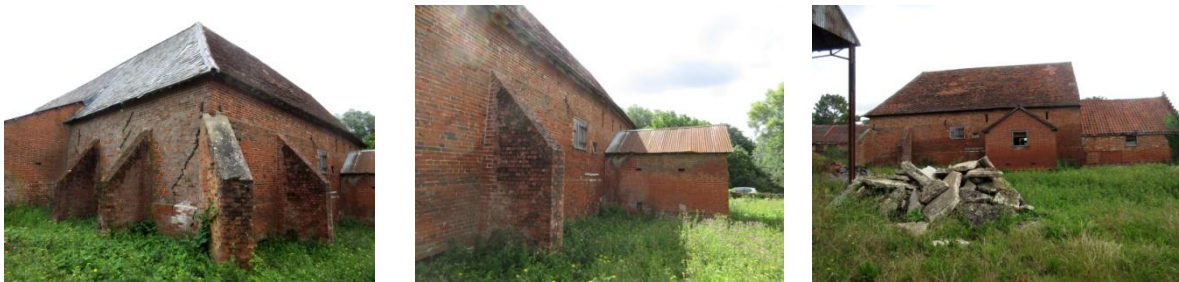
Left: buttresses at NW corner of main barn, looking SE; Centre: looking S showing collar house C attached to W elevation of stable B: W elevation of complex, looking E
