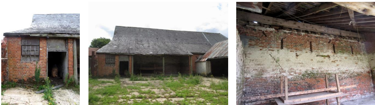
Left: N elevation of building J; Centre: looking S showing 2 open bays of shelter shed I attached to barn A; Right: interior of shelter shed showing ventilation slits and brick dentil course in N wall of barn
