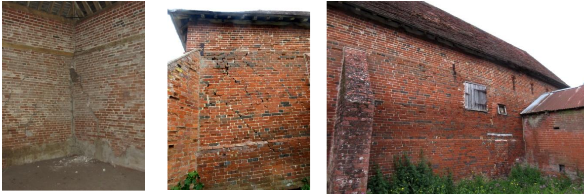
Left: Barn A interior showing settlement cracks in NW corner and changes in brickwork above timber rail where walls were raised in height in the 19th century; Centre: N end of W wall of barn where ground and 1st floor windows are proposed; Right: W wall where glazed double doors are proposed to right of buttress. Loading door to chaff house and smaller opening in stable wall are shown near collar house extension
