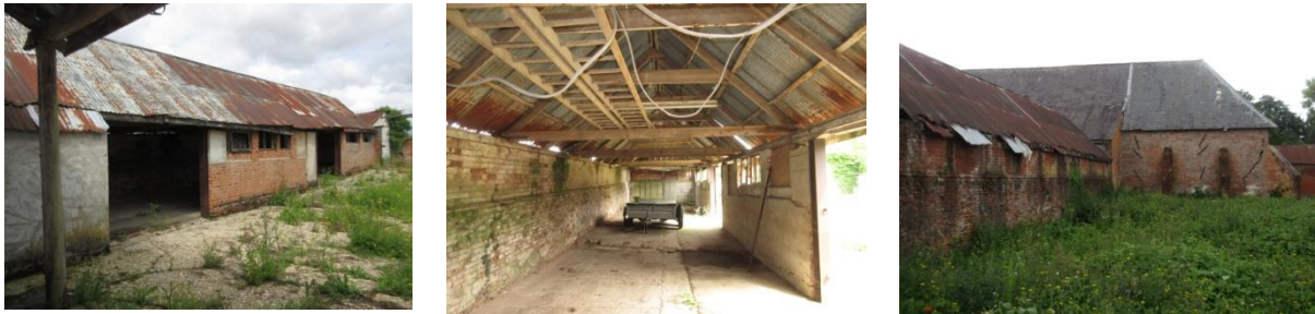
Left: looking NW showing E elevation of milking shed L; Centre: looking N inside milking shed showing W former farmyard wall raised in height in fletton brick; Right: looking S, milking shed on left
