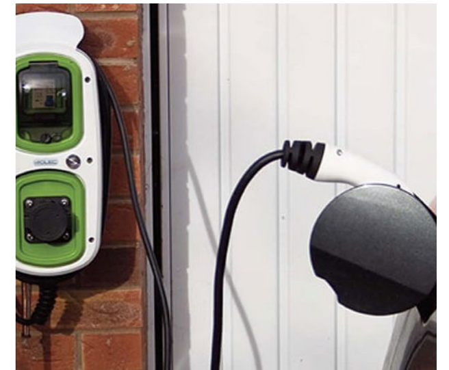
electric car charging points next to all parking spaces
