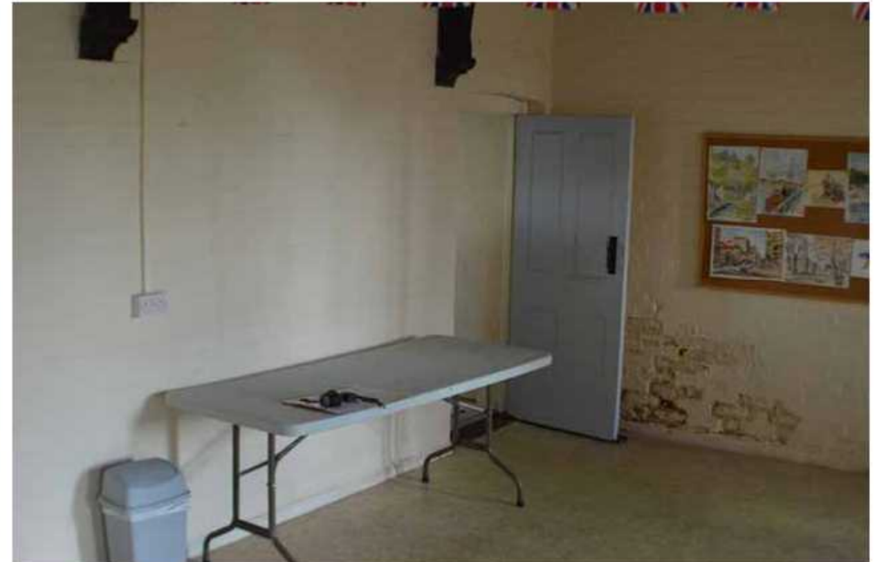
Above: internal photo taken within main hall space existing door through to rear extension, facing north-east.
