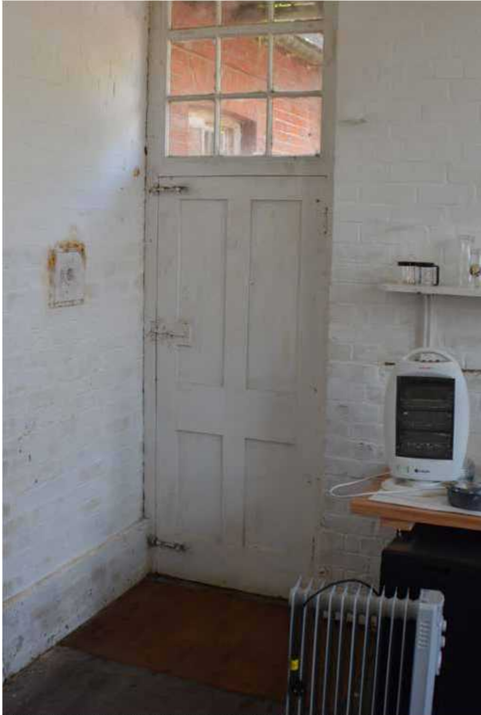
Above: internal photo of timber door located on west wall of rear extension, facing west.
