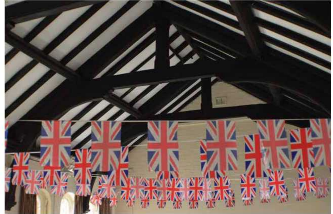
Above: internal photo taken within main hall space illustrating existing vaulted ceiling, facing west.
