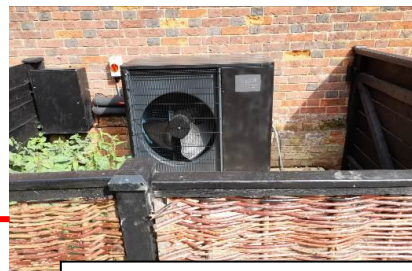
ASHP hidden behind weaved fence
