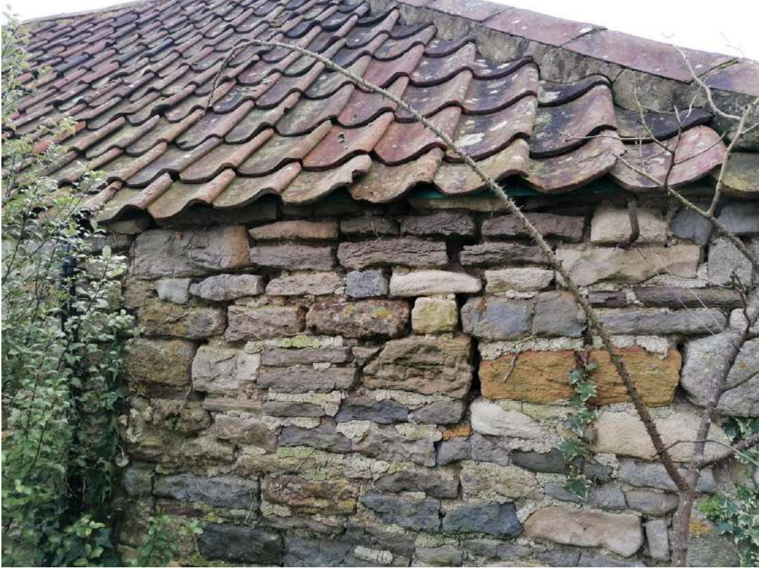
Photograph 8. The east elevation of the Storage Barn showing cracks in stonework (Target Note 4).
