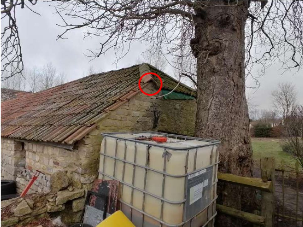
Photograph 7. The east elevation of the Storage Barn showing gaps under ridge tiles (Target Note 3) (circled).
