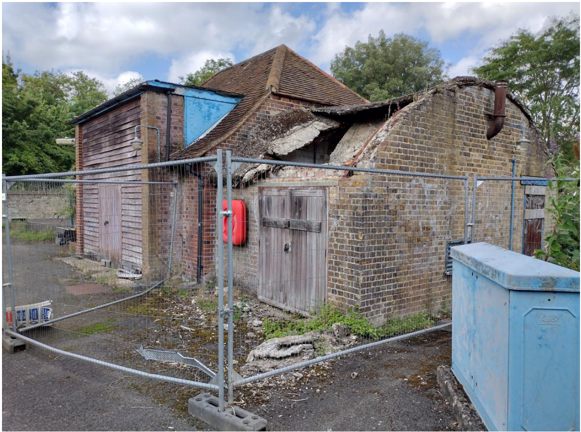
Photo 5: Southeastern elevation showing collapsed concrete roof.
