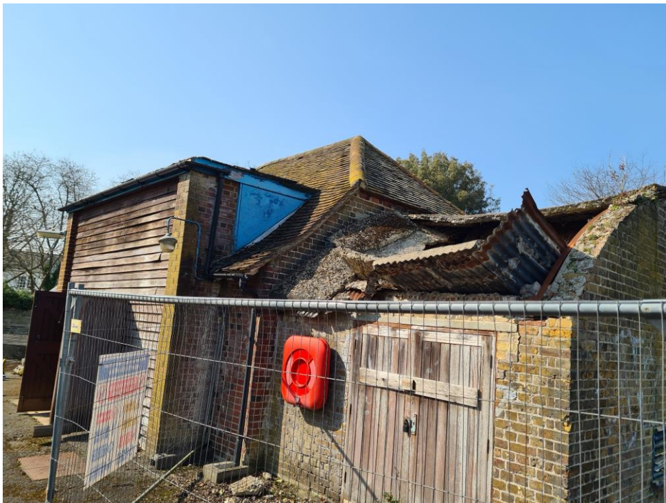
Figure 26: Generator Building collapsed northern roof.
