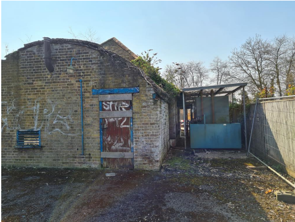
Figure 27: Generator Building in poor state of repair with redundant fuel bunds adjacent to boundary shared with Eton College.
