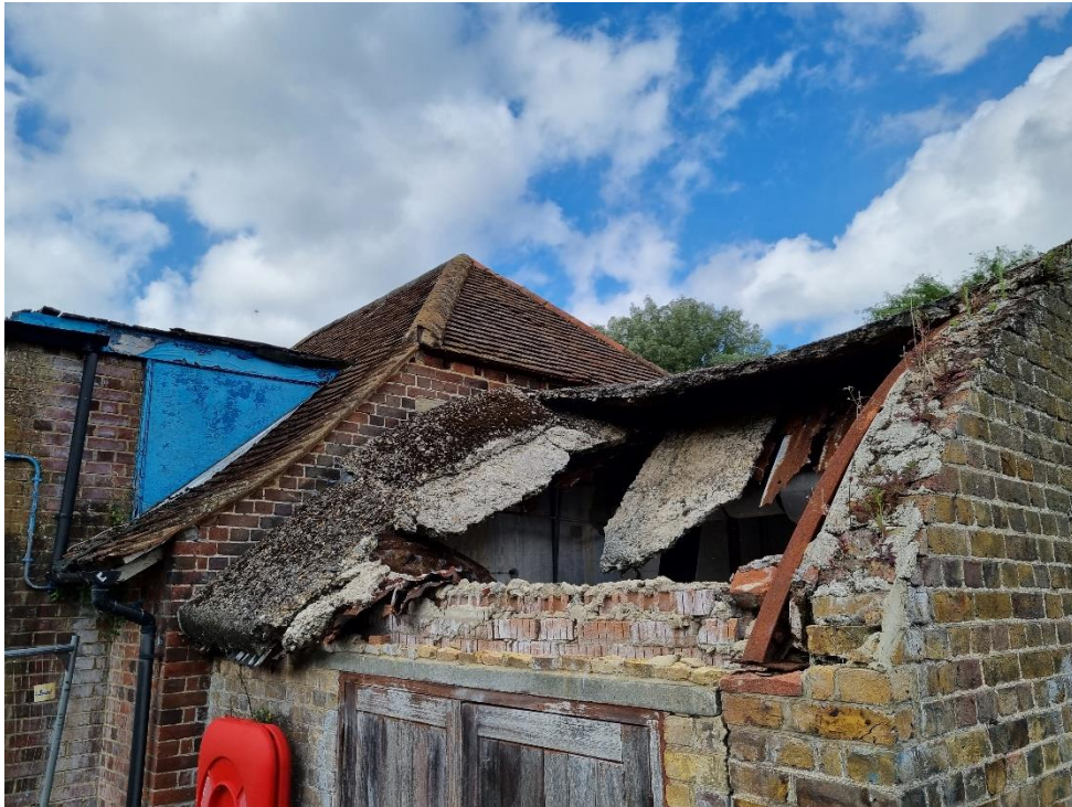
Figure 14: Generator Building collapsed northern roof.
