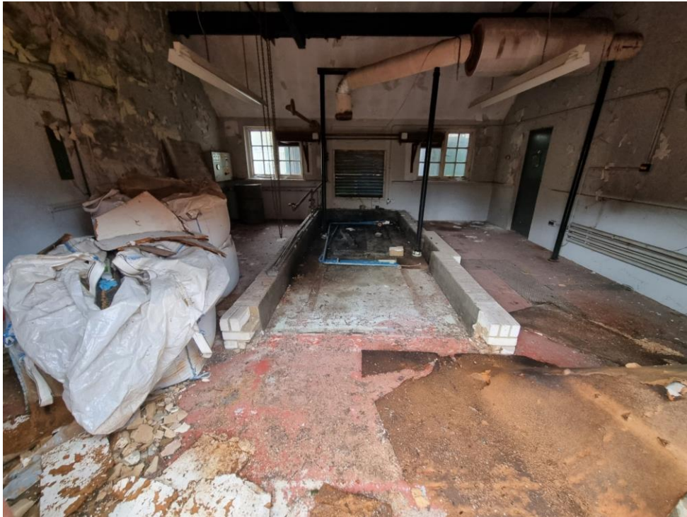
Figure 21: Generator now stripped out.
