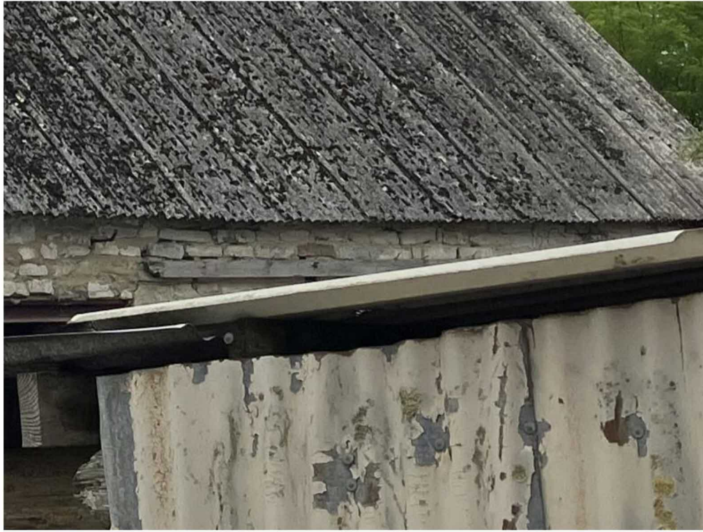
Figure 2 - Asbestos roof sheeting and external images of roof / high level wall structure
