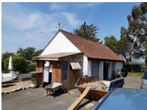
Site Photo 01. Existing South and East elevations of garage viewed from driveway.
