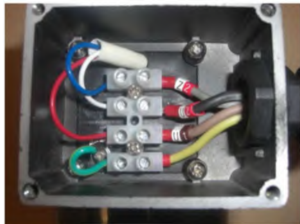
Motor Terminal Box
