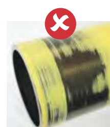
Incorrect pipe preparation for electrofusion
