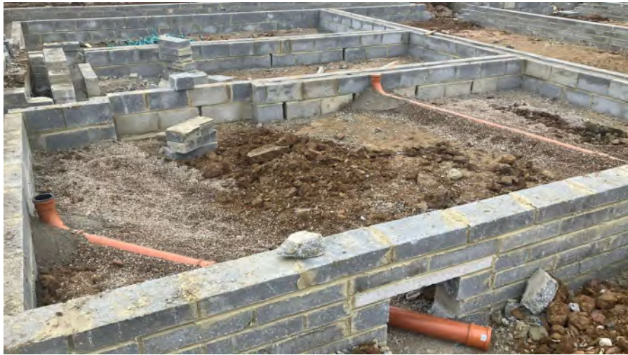
Foul Water Drainage
