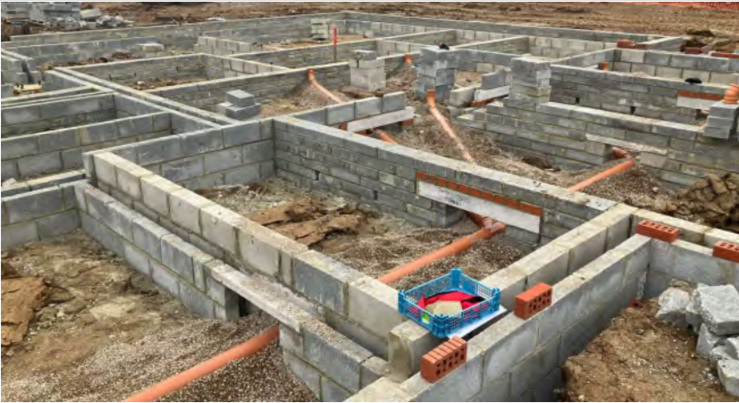
Foul Water Drainage
