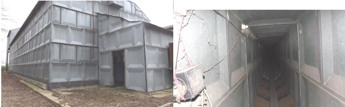
Figure 5 – External view of grain dryer and entrance lean-to at south-west elevation (left), internal view of grain dryer (right)
