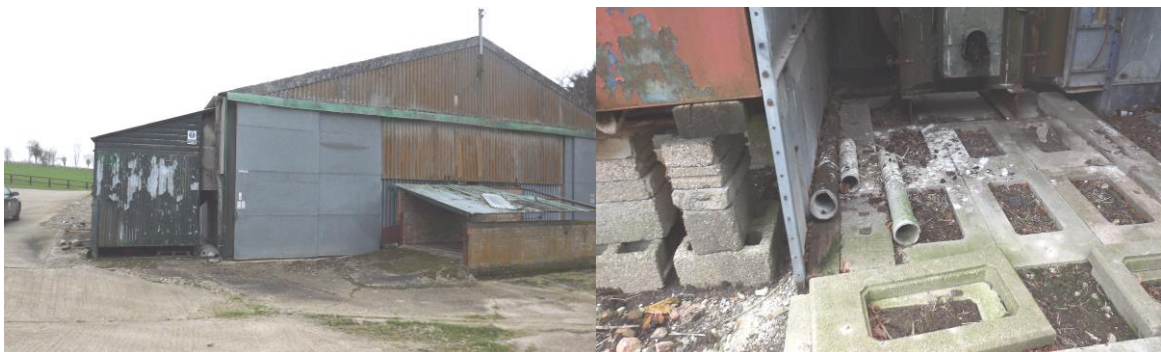
Figure 7 – View of lean-to sections including chemical store, glass house (left) and barn owl use of B2
