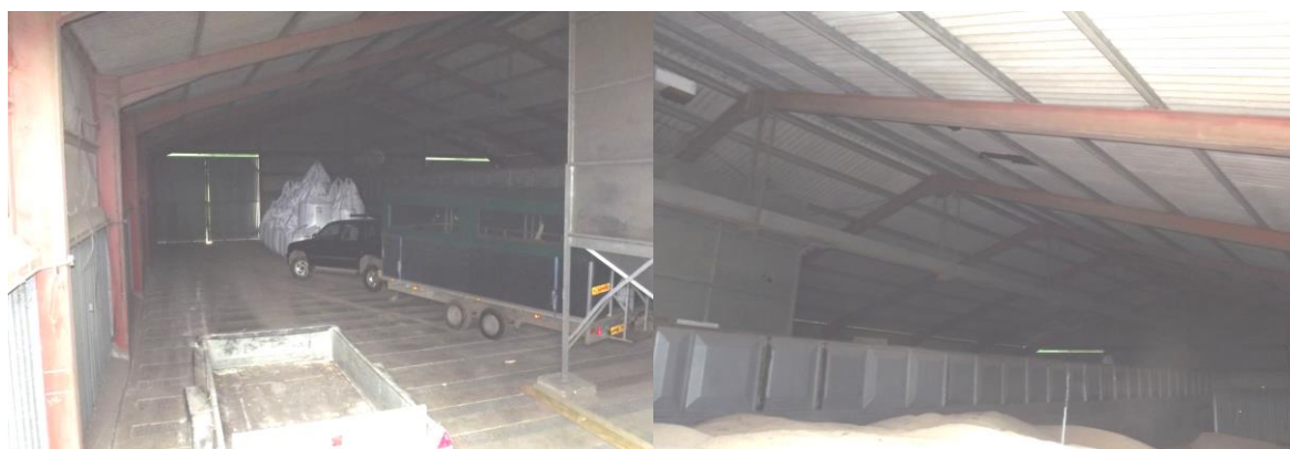
Figure 4 – Internal view of grain store B1 (left), and corrugated asbestos sheet roof (right)
