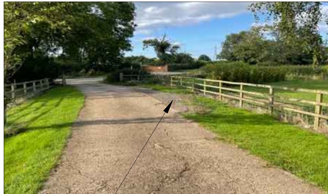
Recently completed widening works (in general accordance with drawing 23529-02). Construction included Type 6F2 base and tarmac planings.
