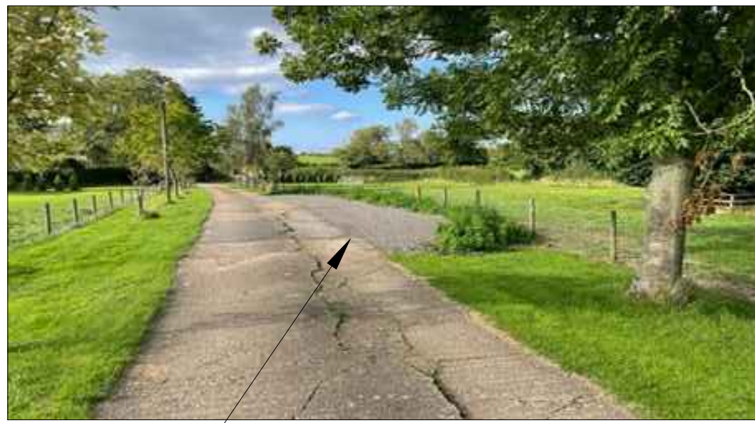
Recently completed passing bay (in accordance with drawing 23529-02). Construction included Type 6F2 base and tarmac planings. To level the passing bays the base was built up to match the existing driveway height and the sides were battered with top soil.
