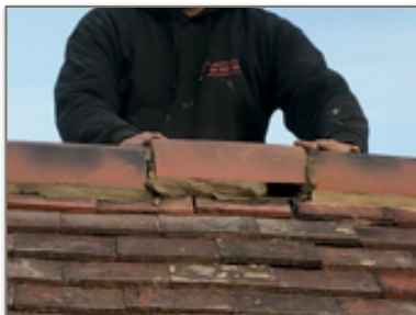
3. Leave the gap mortar free when bedding the tile onto the ridge.
