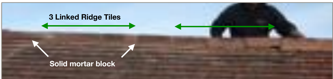
5. At each end of the three linked ridge tiles insert a solid mortar block to reduce through draughts.
