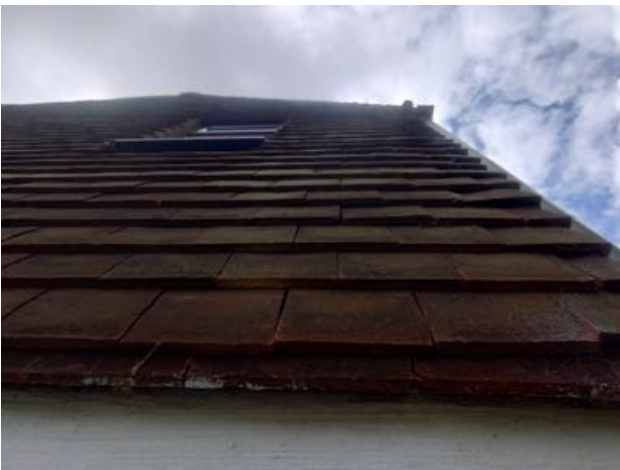
Image 3: The hanging tiles on the north elevation which will be impacted by the works.
