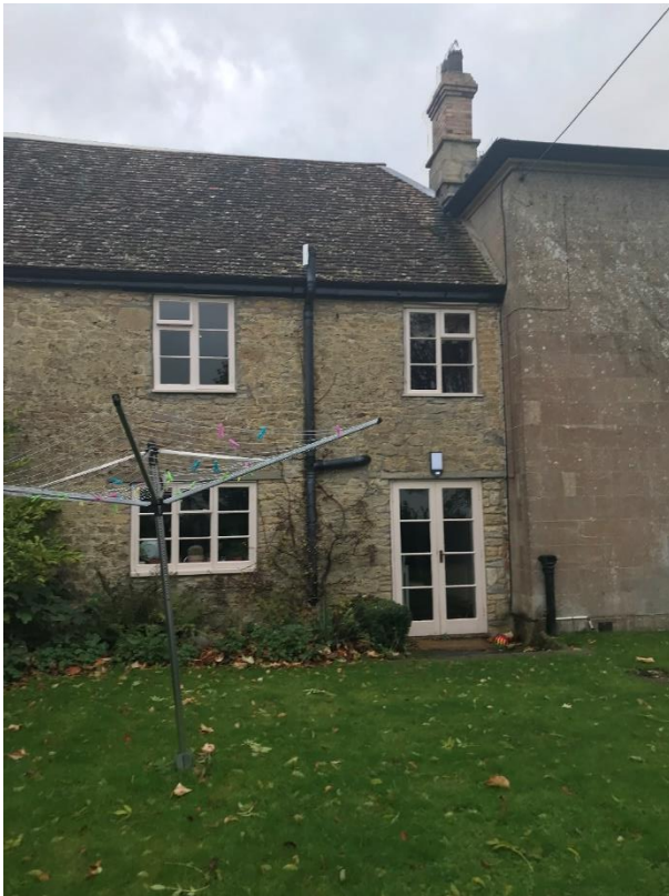
Figure 20 – The front 19 th century range is formed of ashlar which contrasts to the rubblestone of the original range.
