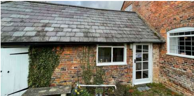
South elevation - The barn door and window to be removed and replaced with double doors
