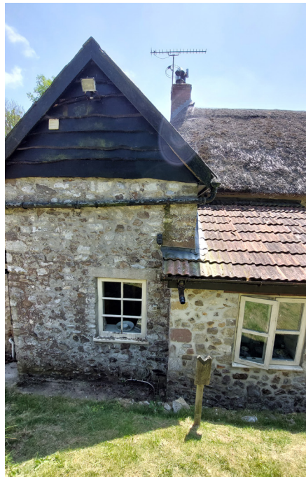
Figure 8 - Window to be adapted to form a new opening to the proposed extension
