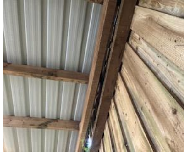
Photo 2: Large gaps between timber frame.
