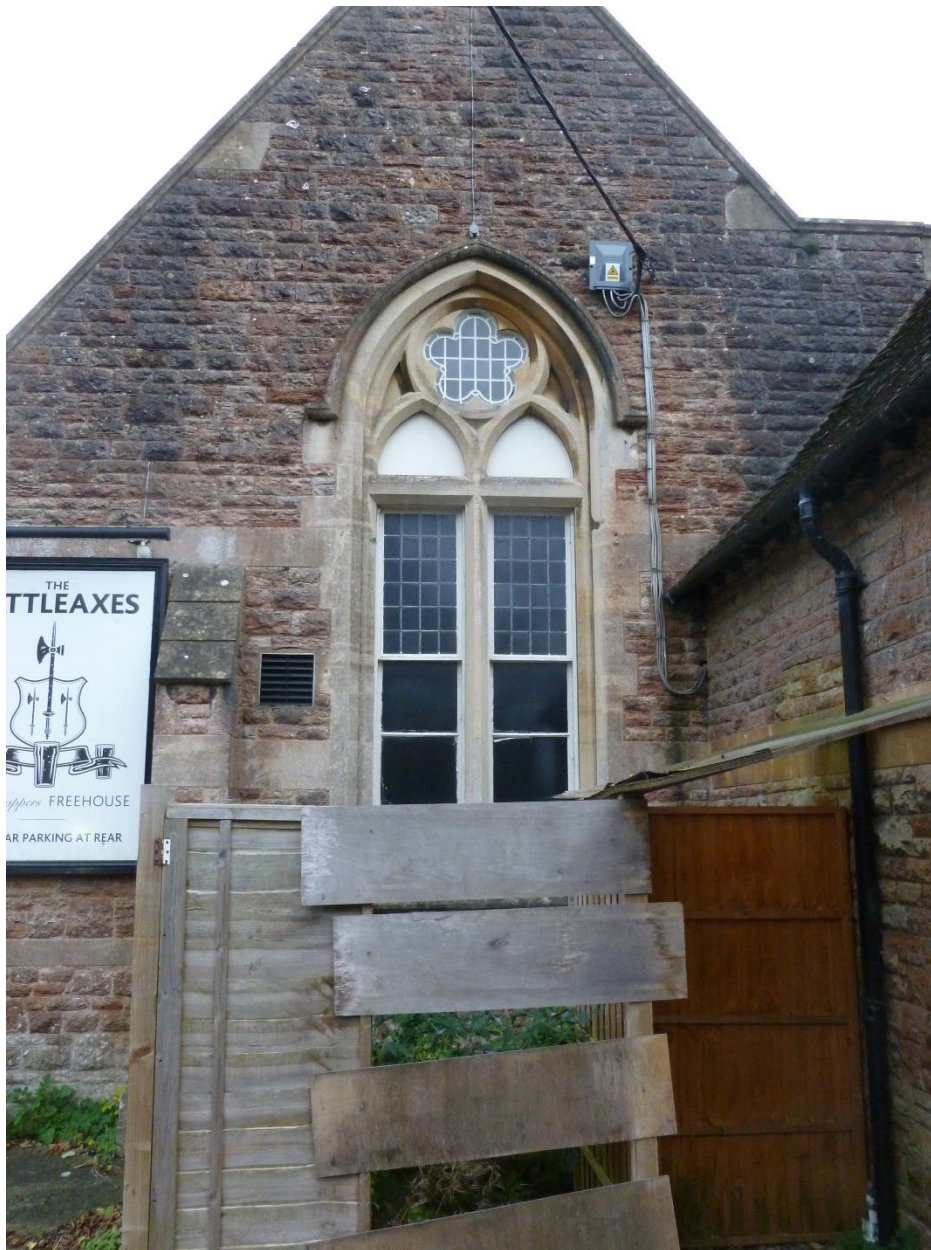
Plate 11: Blocked western window to the Hall
