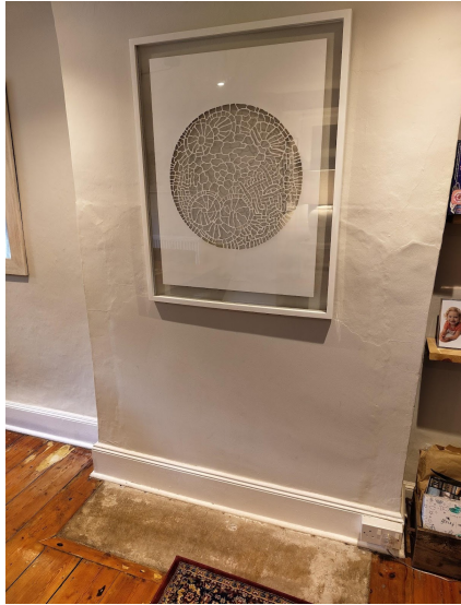
Photo shows blocked fireplace in the dining room with the original hearth.
