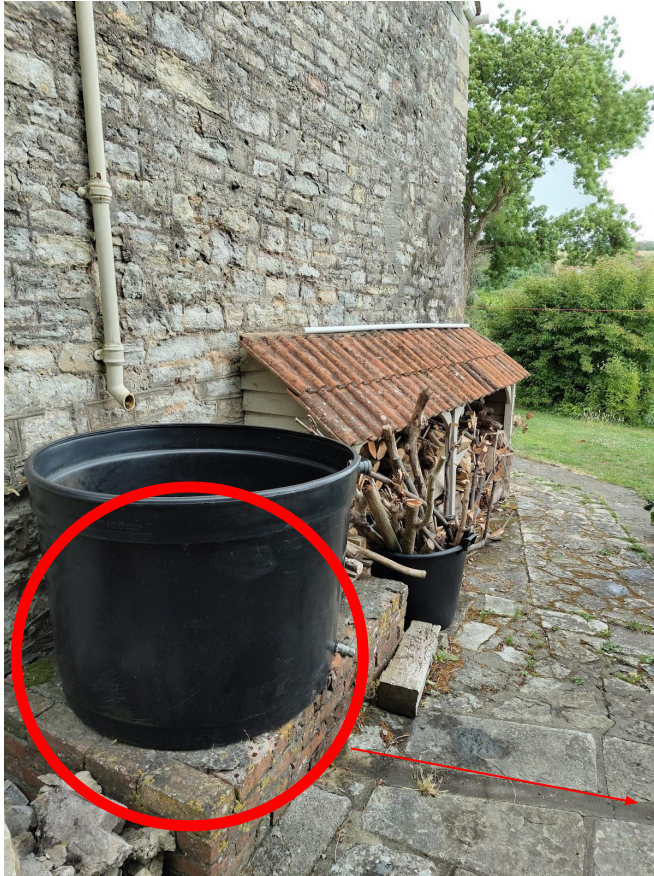
Photo showing old water butt with degrading brick base and outflow.
