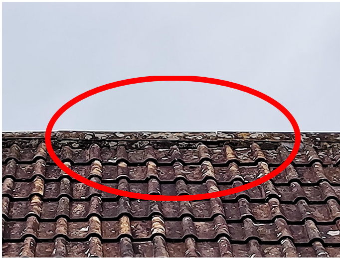
Photo showing bedding mortar failure
