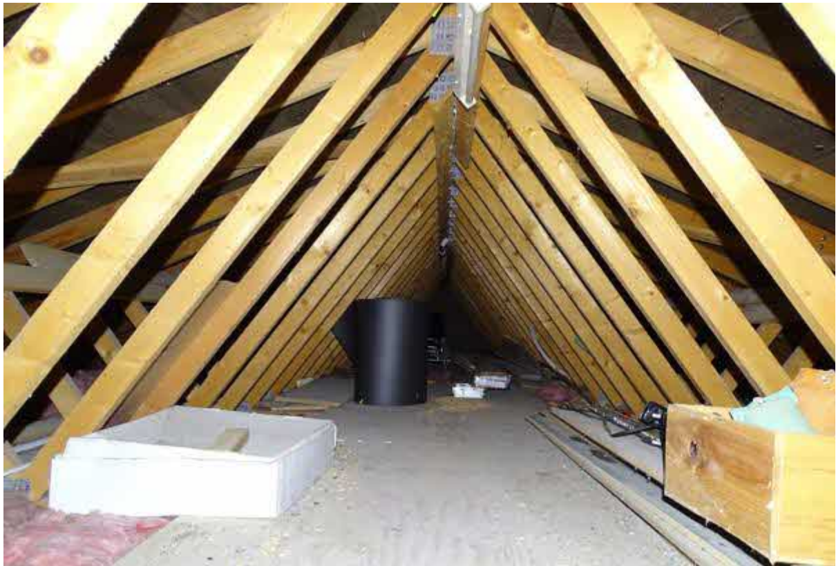
Image 17 – Building two – Internal view from within the inner roof void spaces of the building
