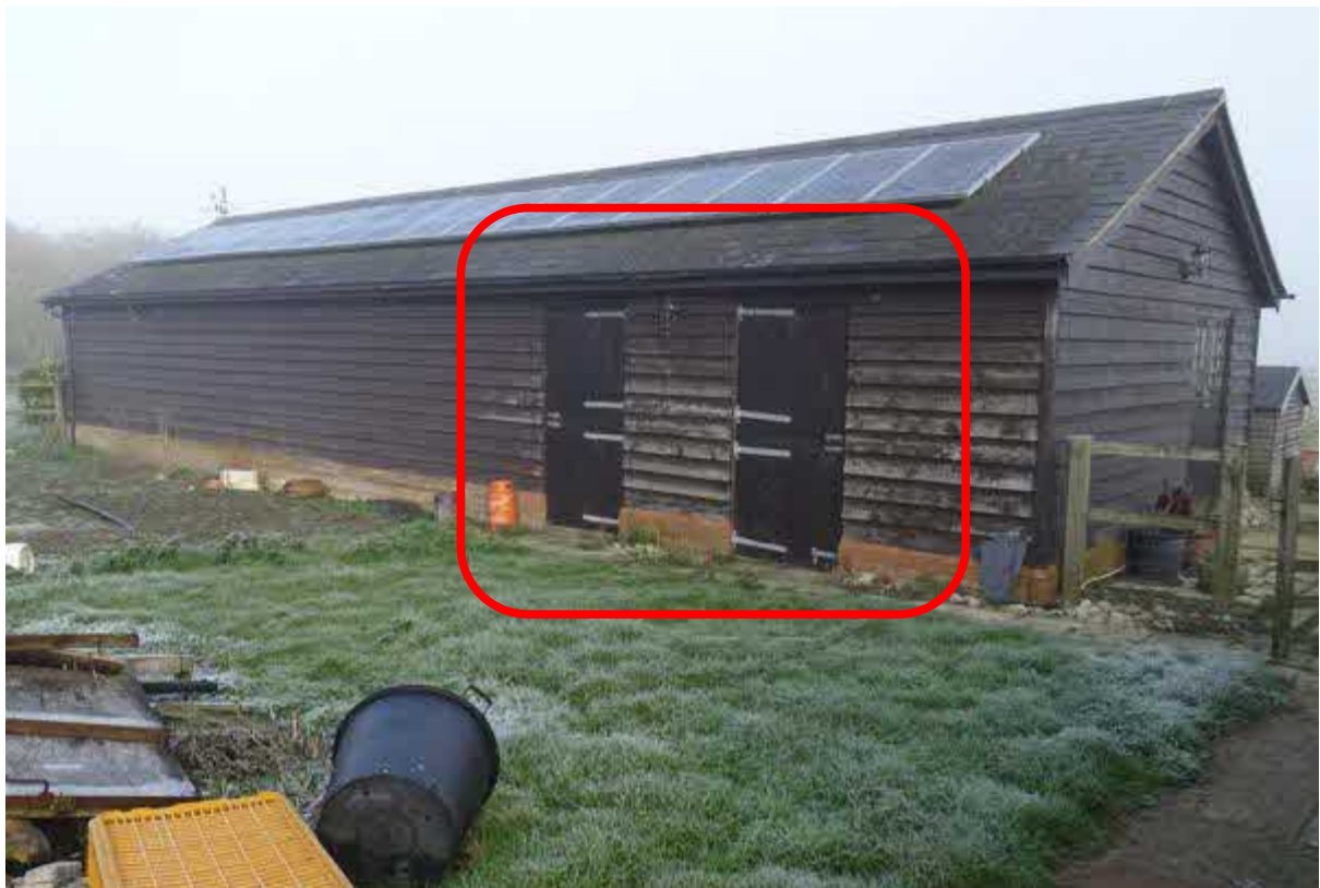
Image 14 – Building one – South/West facing elevation of the building which has evidenced gaps around the timber doors
