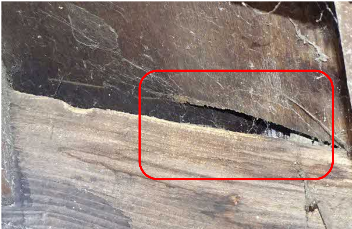
Image 16 – Building two – Small number of gaps within the eaves areas of the building which look to offer further likely shelter/access opportunities for bats
