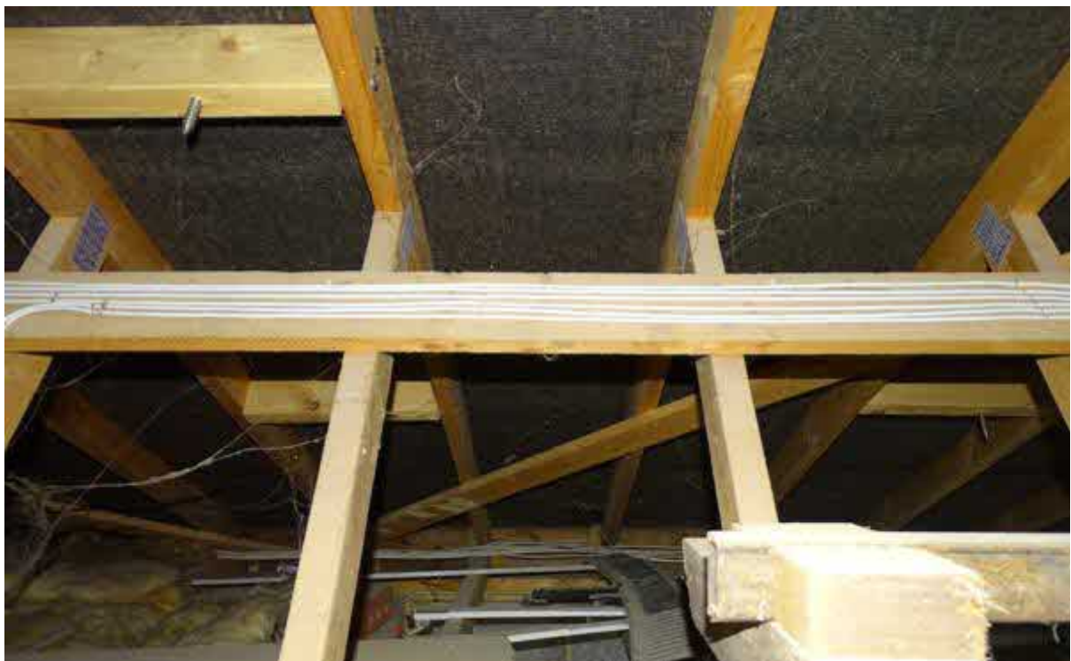
Image 18 – Building two – Internal view from within the inner roof void spaces of the building
