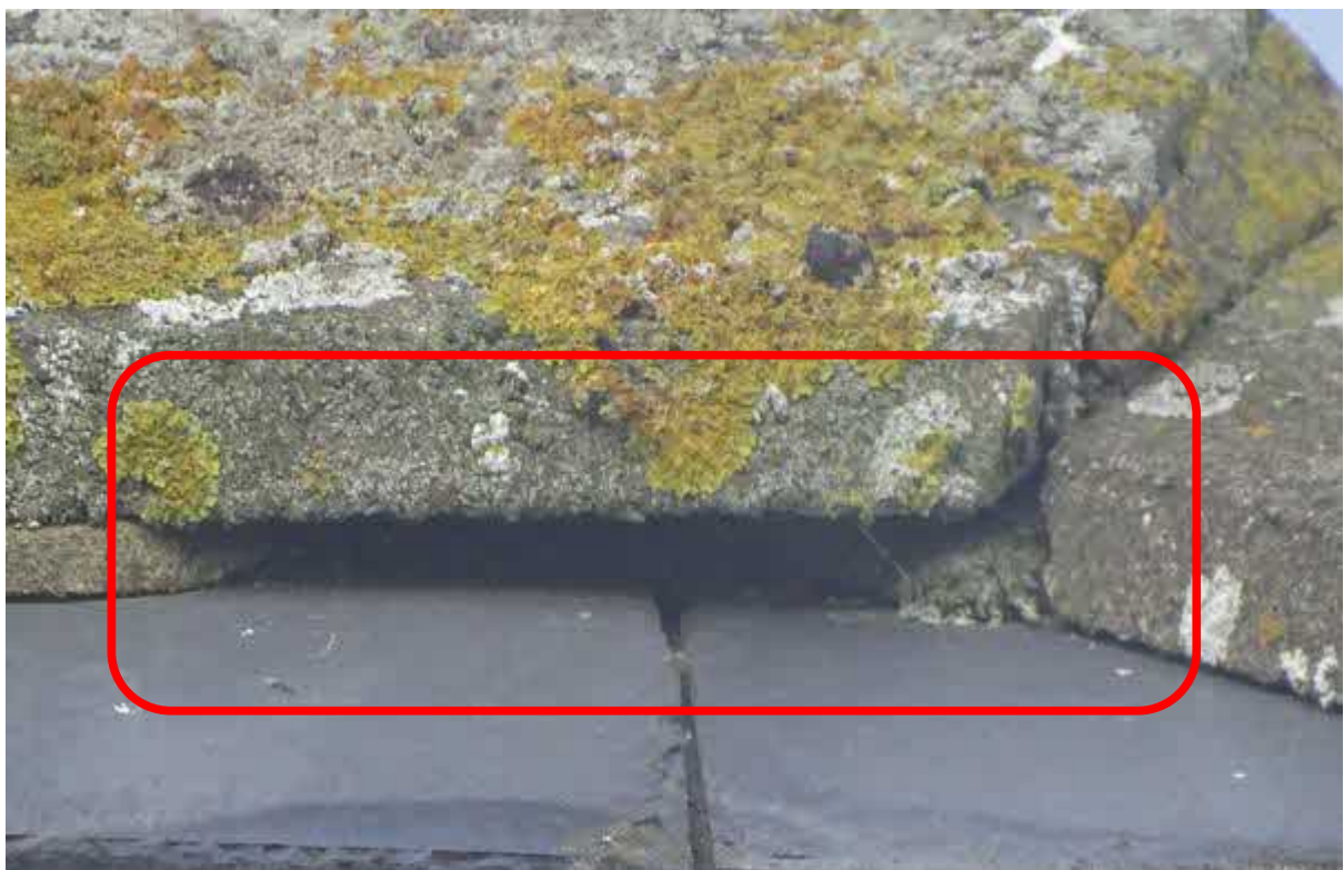
Image 10 – Building one – Gaps observed below the ridge coverings offering further shelter/access opportunities for bats within
