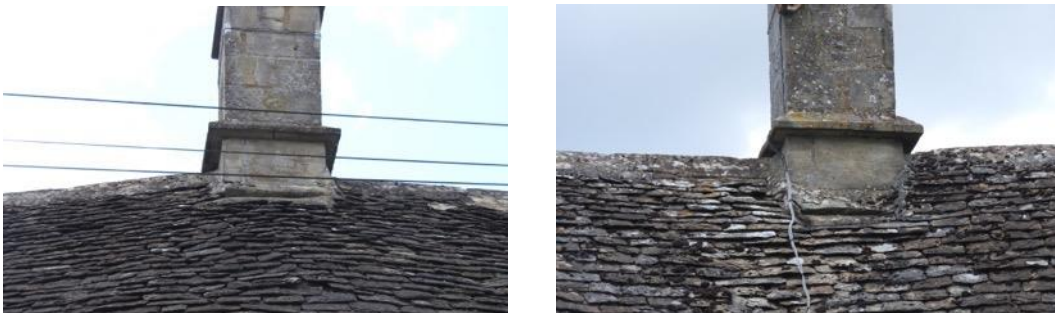
Figs. 11 & 12 Sealed chimney bases
