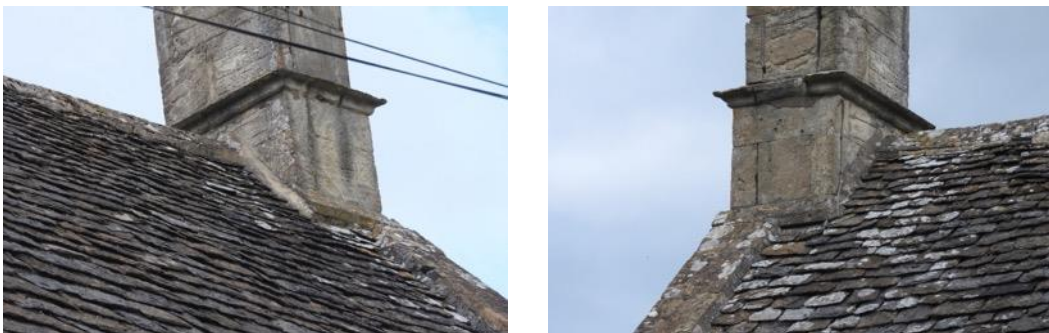
Figs. 13 & 14 Sealed chimney bases
