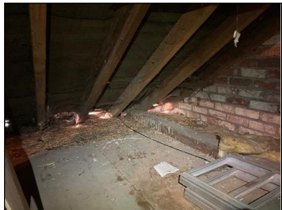
Plate 6: Gaps at eaves level & bird nest material
