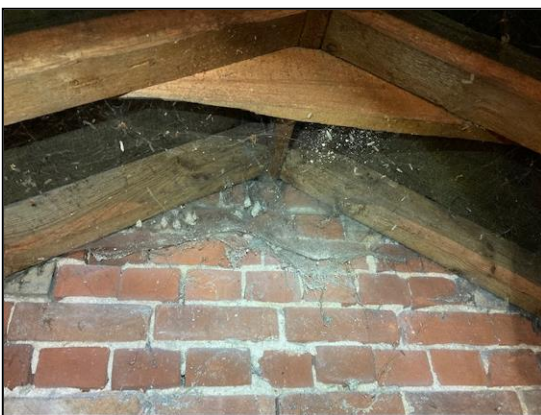
Plate 11: Cobwebs at roof apex
