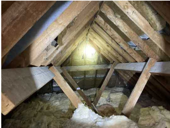
Photograph 9: Example of roof with degraded membrane
