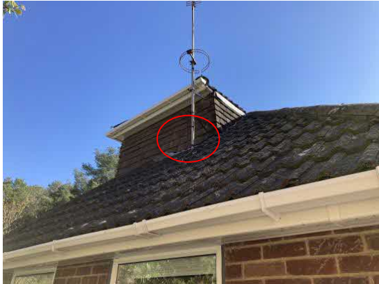
Photograph 7: Missing tile behind satellite dish
