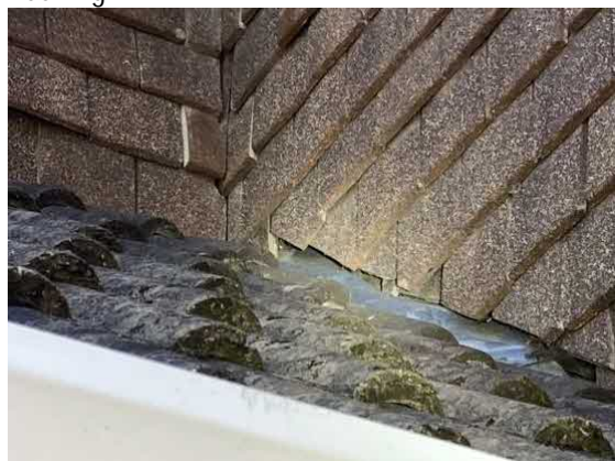
Photograph 6: Gap between hanging tiles and lead flashing
