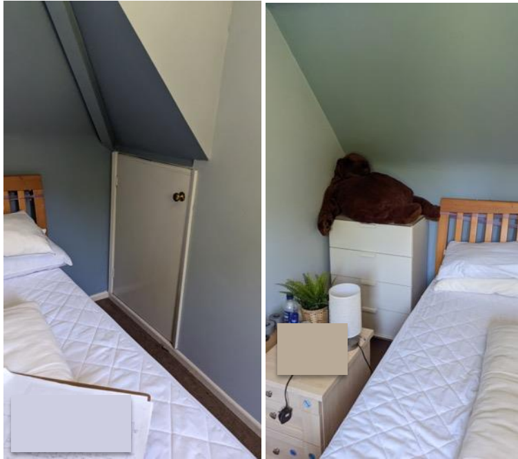
Images 10 & 11: Showing reduced headroom to first floor bedroom.
