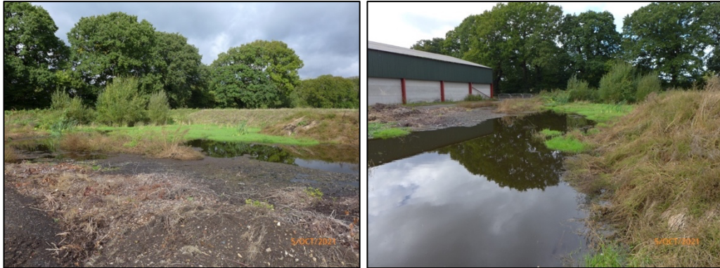
Figures 4 & 5: Disturbed ground and standing water between western earth bank and grain store
