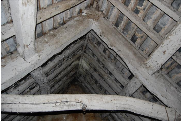
Photograph 7. Heavily cobwebbed underside of the roof of the attic room (third floor).
