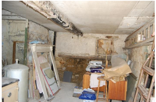
Photograph 4. The eastern-most garage/storage room, with stairs (in the back left corner of the room) leading to the first floor.
