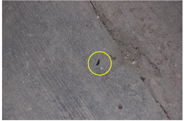
Photograph 8. Brown long-eared bat dropping on the floor of the north-western first floor room (outlined in yellow).
