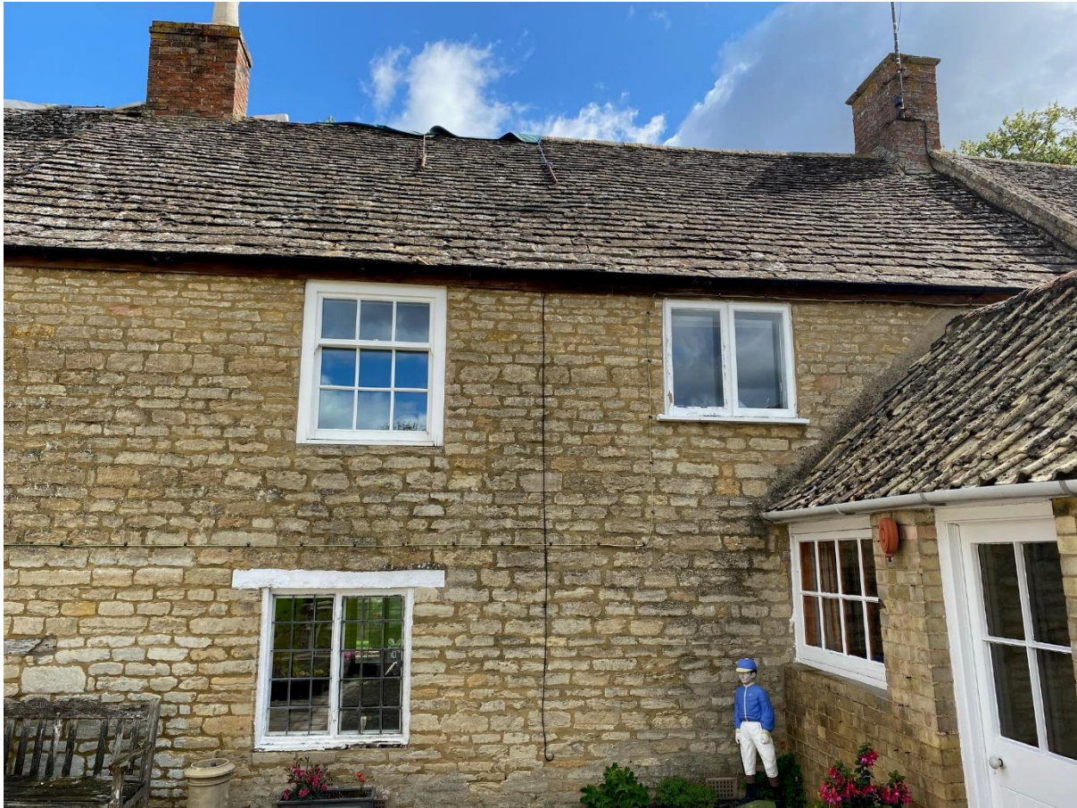
Fig 7 First floor sash and casement windows to be replaced with leaded windows to match original cottages
