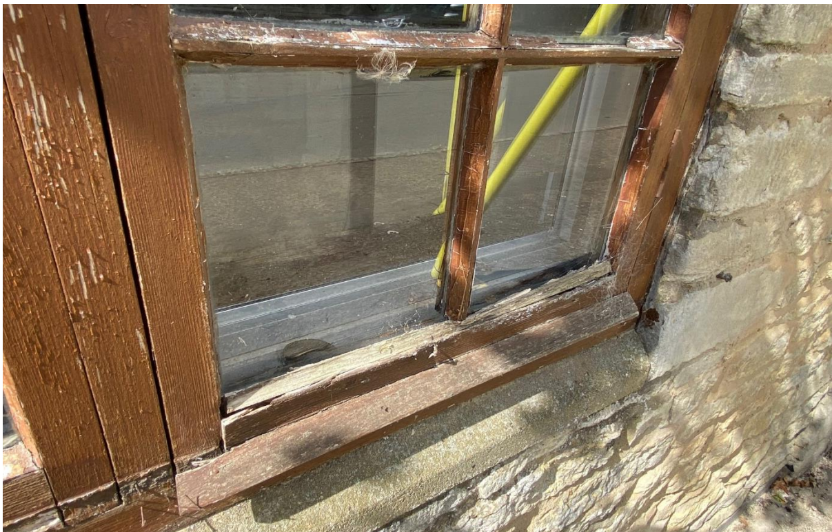
Fig 6 Poor condition of existing dark stained single glazed windows in “newer” cottage
