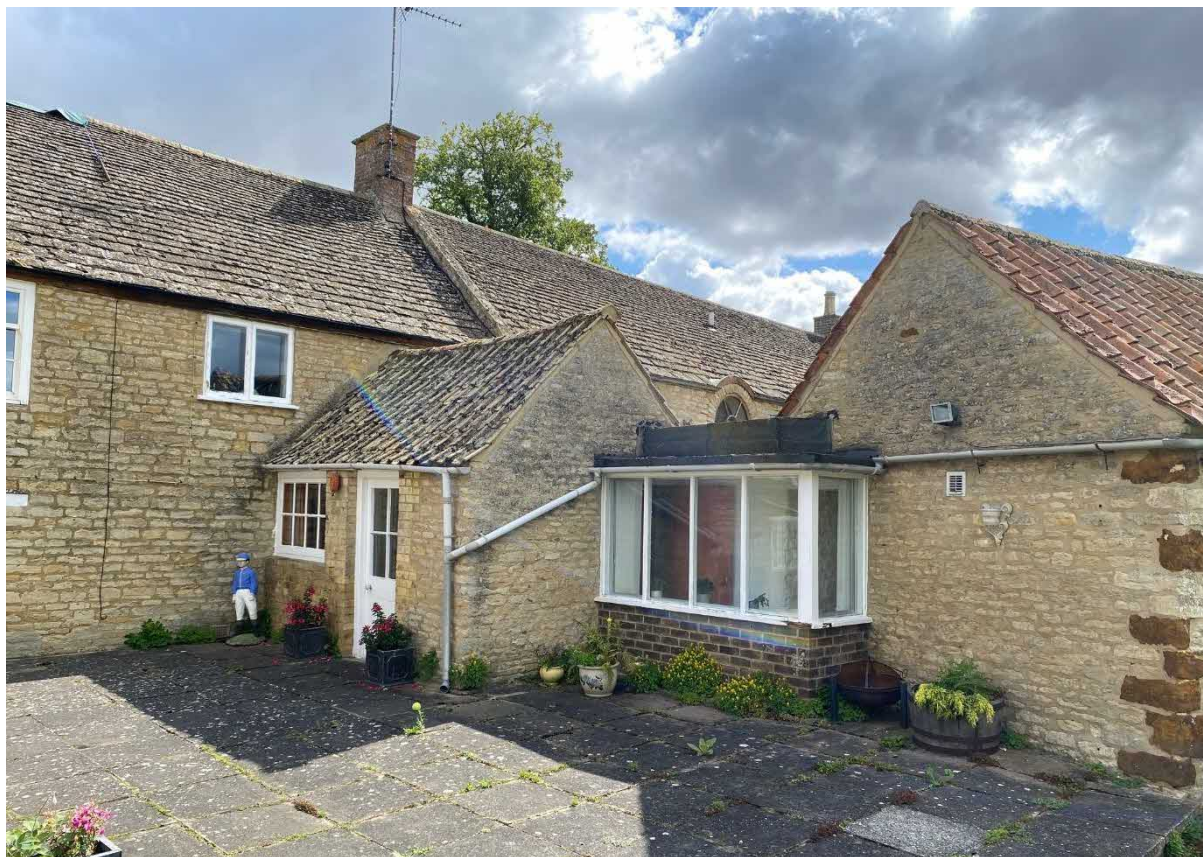
Fig 4 Current link structure to be demolished, note first floor casement windows to be replaced
