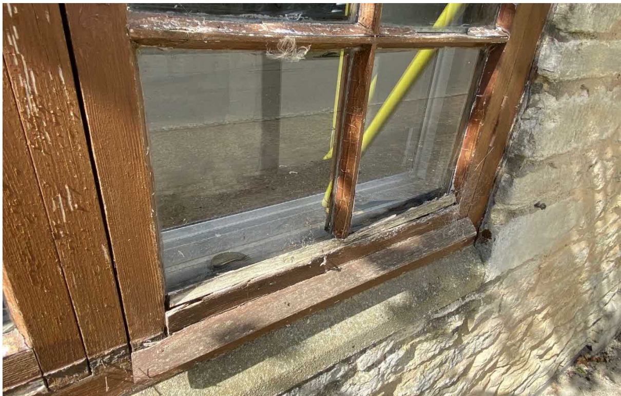
Fig 6 Poor condition of existng dark stained single glazed windows in “newer” cottage
