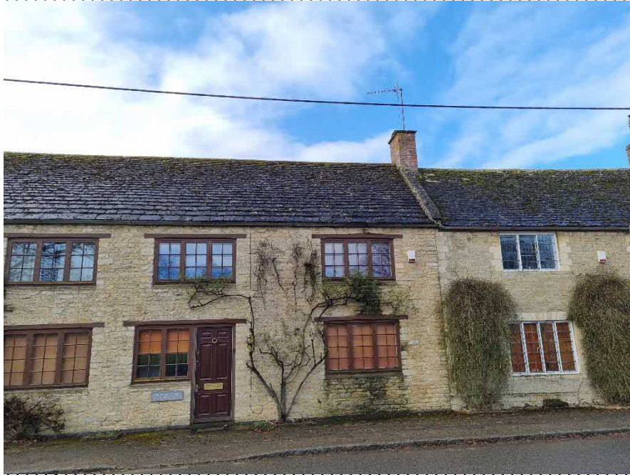
Plate 3. Deterioration due to defective gutter.
