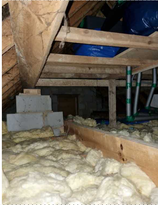
Plate 17. Minor disruption at wall plate.
