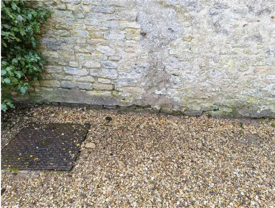
Plate 9. Accelerated weathering due to lack of gutter above
