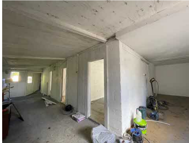
Photograph 20a: View of Section B interior with inaccessible roof void above in 2023.
