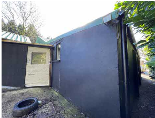
Photograph 13: View of the north elevation of Section C with Section E walkway to the left.
