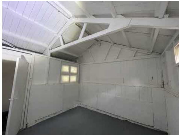
Photograph 24a : Section D interior with timber sarking boards lining the roof in 2023.
