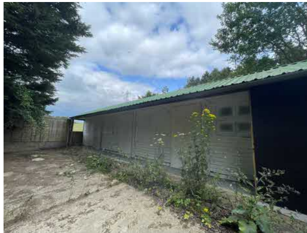
Photograph 22b: New porch area along west elevation of Section D where boarded walkway had been removed.
