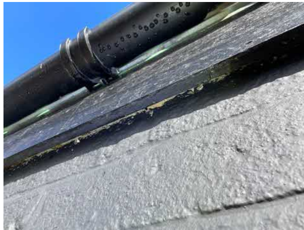
Photograph 17: Gap behind the timber fascia board of Section A.
