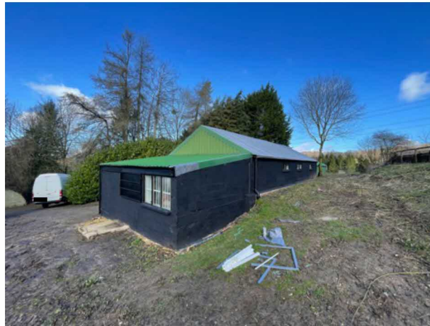
Photograph 11: View of Section A lean-to attached to the gable end barn, Section B.
