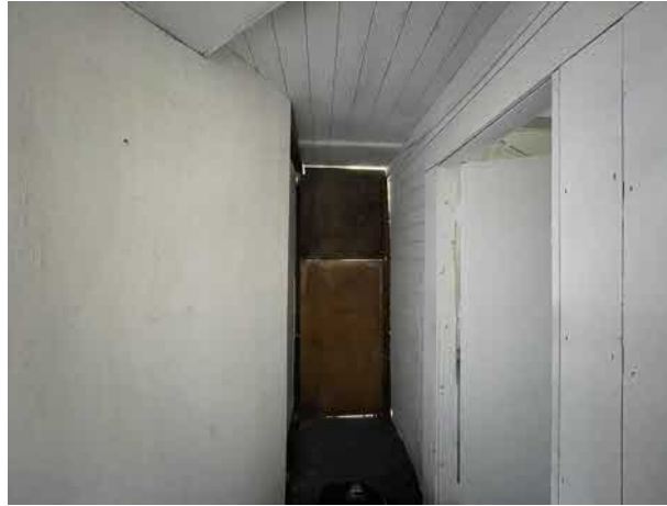
Photograph 22a: Walkway along west elevation of Section D had been sealed off.
