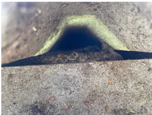
Photograph 23: Gaps along the corrugated roof of Section D.
