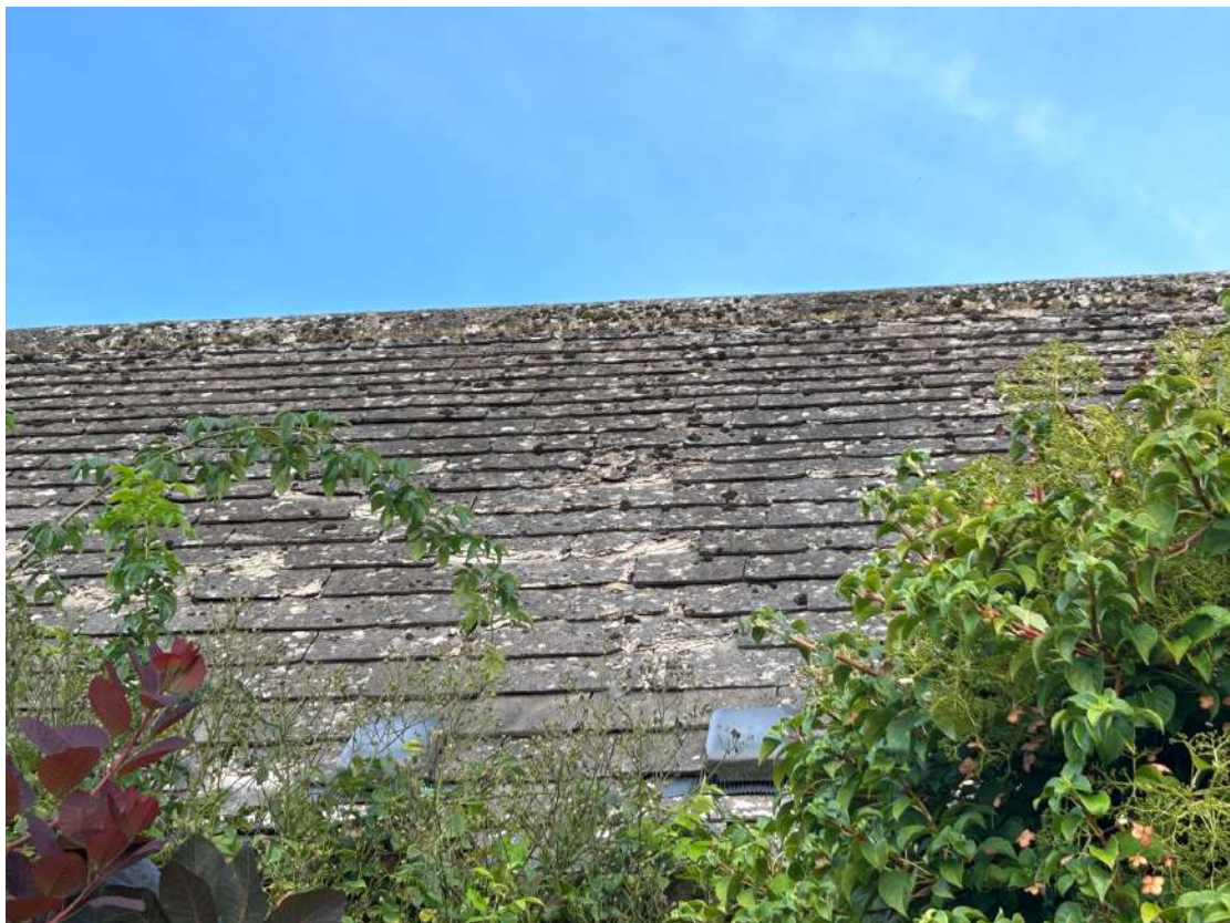
Above: Delaminated slates
