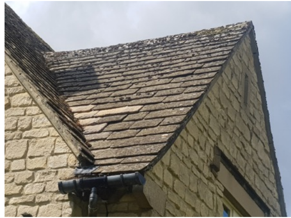
Photo 2: B1 - Raised tiles
