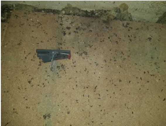
Photo 7: B1 - Scattered bat droppings on floor of loft
