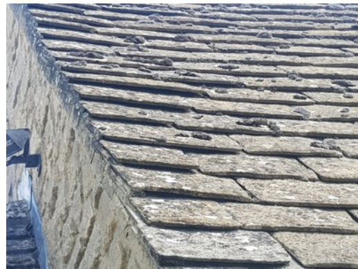
Photo 10: B2 - Raised tiles
