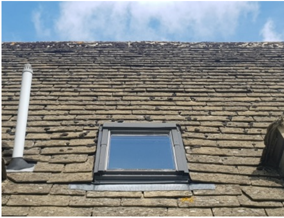
Photo 73: B3 - Raised tiles
