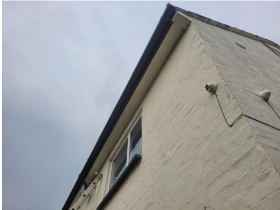
P3: Example of the tightly soffited eaves
