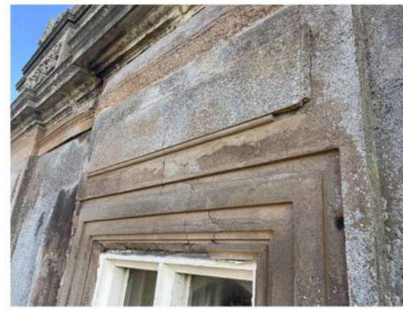
4- Cracked render to window surround & loss of moulding
