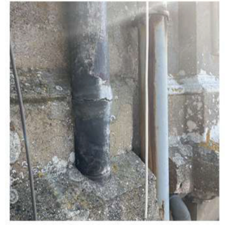
11- Defective render to reveal above cill
