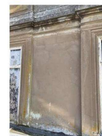
17- Extensive map cracking to flat render panel
