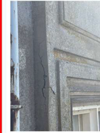
9- Extensive cracking to window reveal
