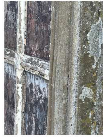
6- Cracking to render at reveal
