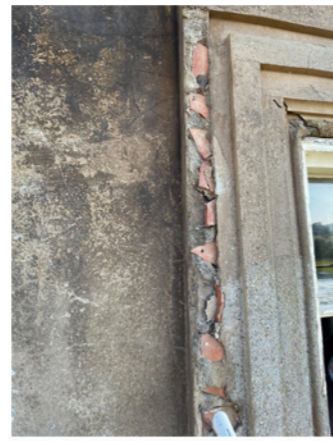
2- Failure of render to built up reveal
