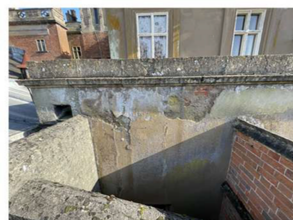
18- Defective flat render to parapet and light well
