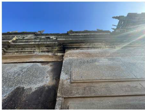
1- Open joints to cornice
