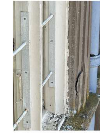
10- Defective render to reveal above cill
