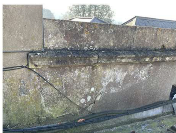
12- Cracking to render to external side of parapet
