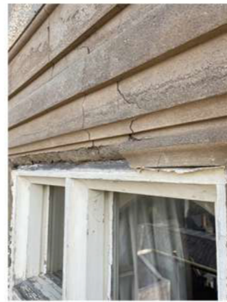
3- Heavily cracked render to window head
