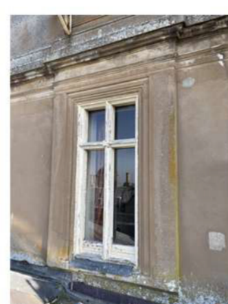
14- Cracking to render at base of window surround & entablature
