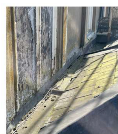
13- Cracking through false window & render reveal
