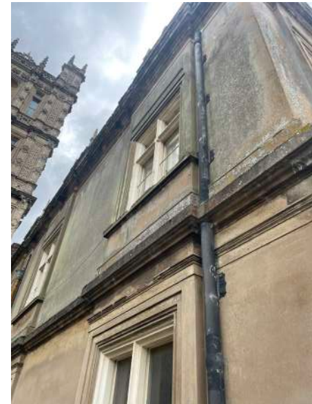
Fig. 28 The adjacent rendered wall that faces North to meet the central tower.
