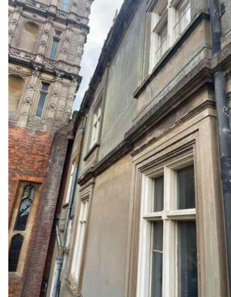
Fig. 26 The adjacent rendered wall that faces North to meet the central tower.
