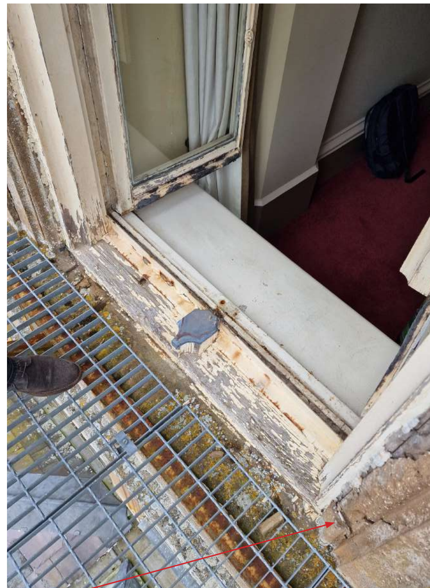
Fig.15. (Above) The second floor gantry egress window. The red arrow indicates where the loose render sample originated from, to the right hand side of the window reveal.
