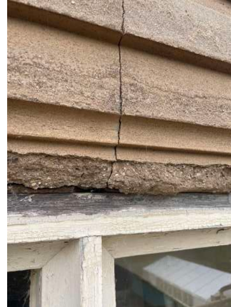
Fig. 30 Fissure cracks in the decorative render.
