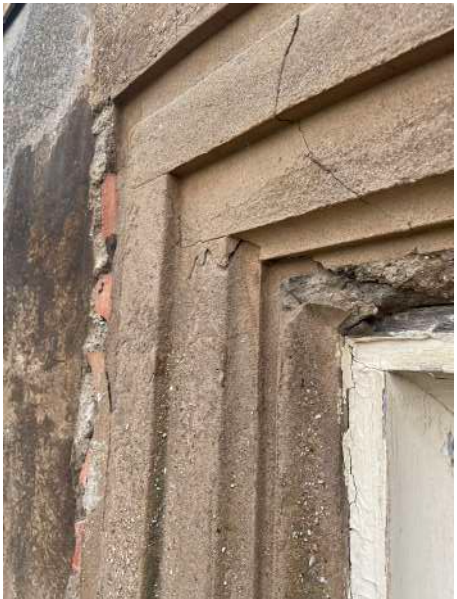
Fig. 31 Fissure cracks emanating from the corner stress lines.
