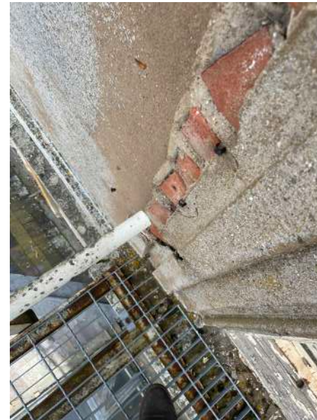
Fig. 32 Collapse of the render face to reveal the clay tile fragments used as packers.
