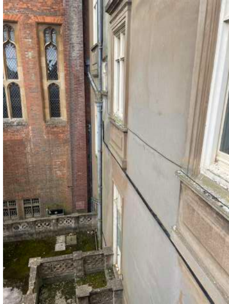
Fig. 25 The adjacent rendered wall that faces North to meet the central tower.
