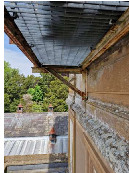
Fig. 34 The poor condition of the gantry steelwork decorations.
