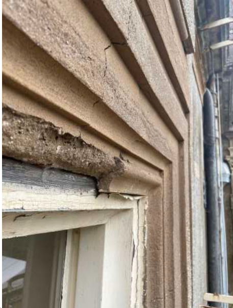
Fig. 29 An example of render falling around the gantry window head.
