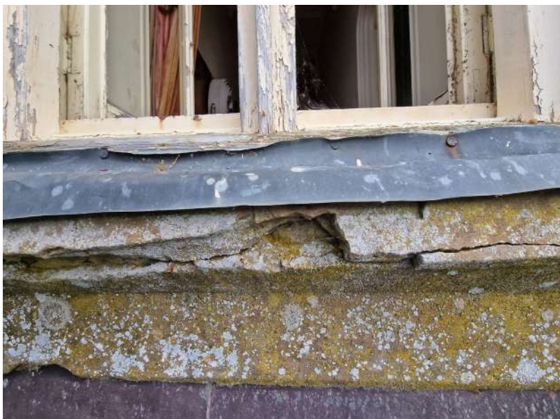
Fig. 35 The falling render flashed below the roof egress window to the first floor
