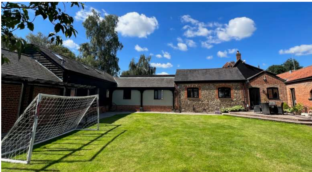
Existing roof-lights (proposed for replacement with conservation-style units) face onto the site’s domestic rear garden where they are discreetly enclosed - and screened from public view - by the dwelling’s U-shape
