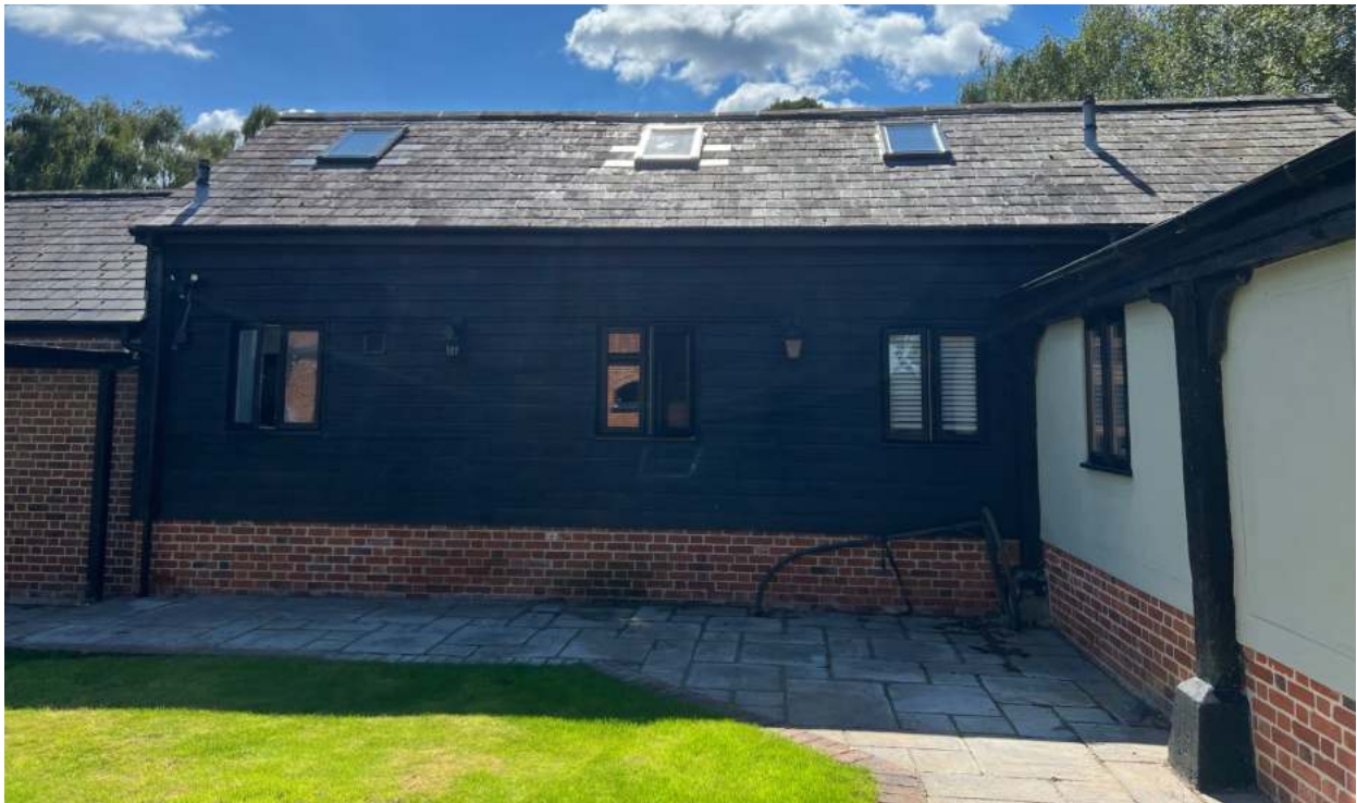
The existing roof-lights in situ, proposed for replacement with low-profile, conservation type roof-lights
