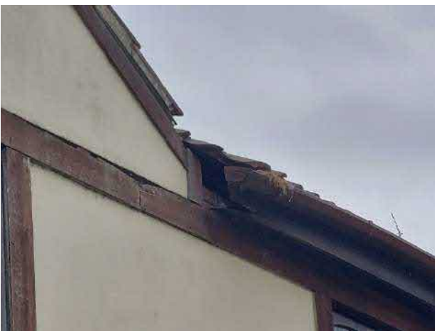
Figure 5. Gap in eaves of B1
