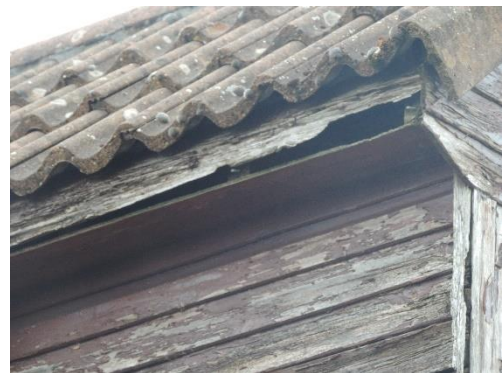
Plate 4: Damaged Soffit Box
