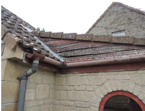
Plate 3: Damaged Weather Boards
