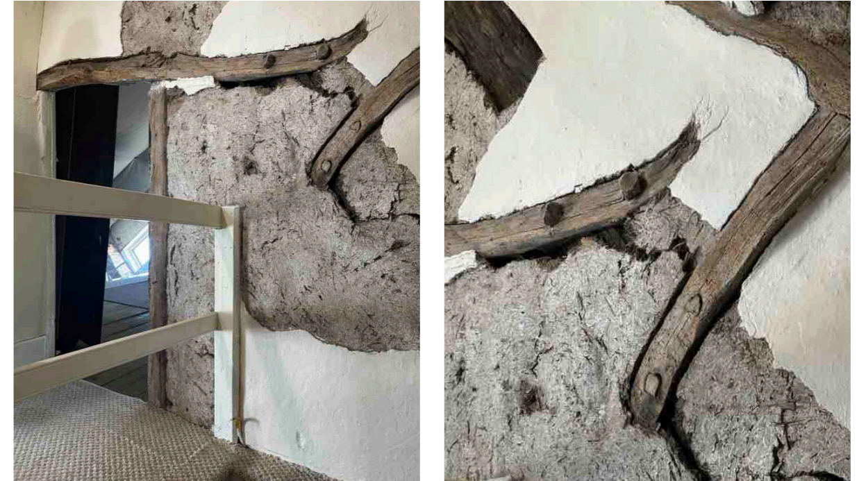
01. View of damage caused due to existing roof weight
