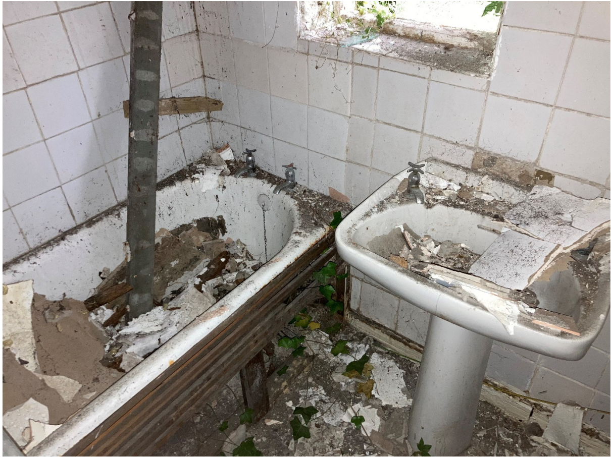
View of existing bathroom (with plaster debris from collapsed ceiling)
