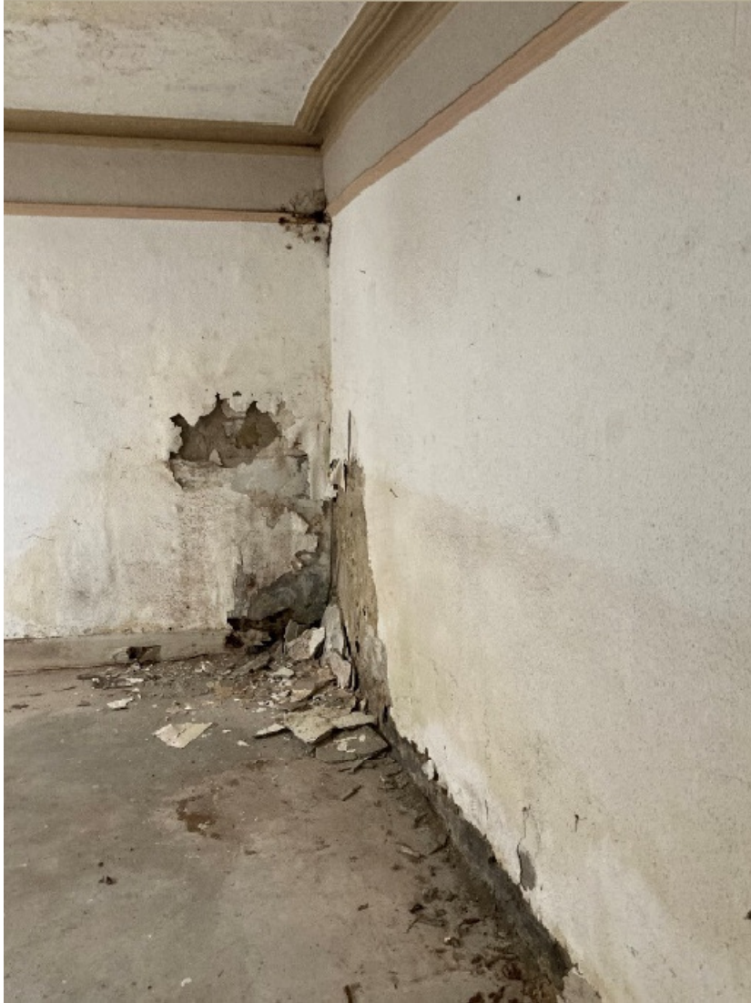
Interior view illustrating rising damp to living room walls
