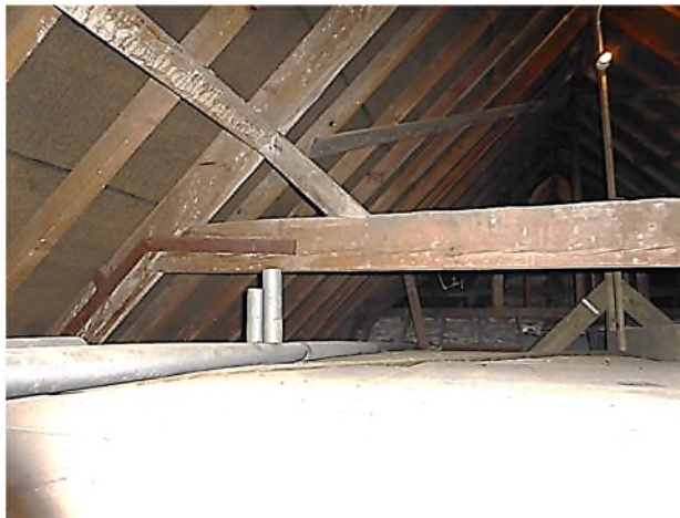
Figure 15: Collar beam truss in the roof void over the central part of the building (2018)
