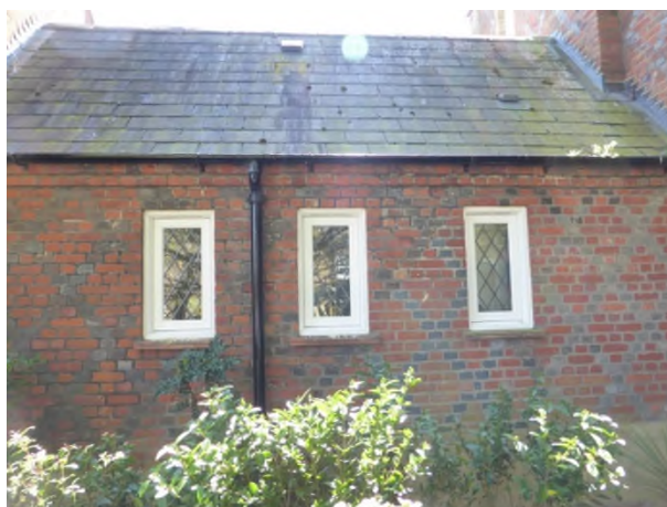
Figure 12: 20 th century window openings on the northern side of the former Closets (G9-G10) (2018)
