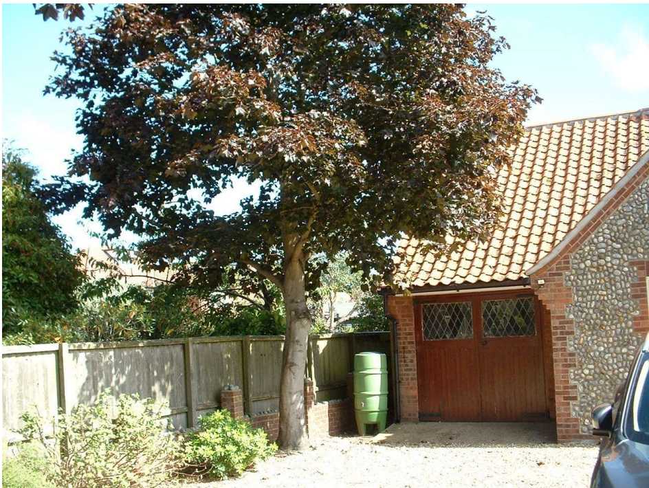
Tree labelled 3(2) showing overhang on roof and location to the bungalow and damage to garden wall
