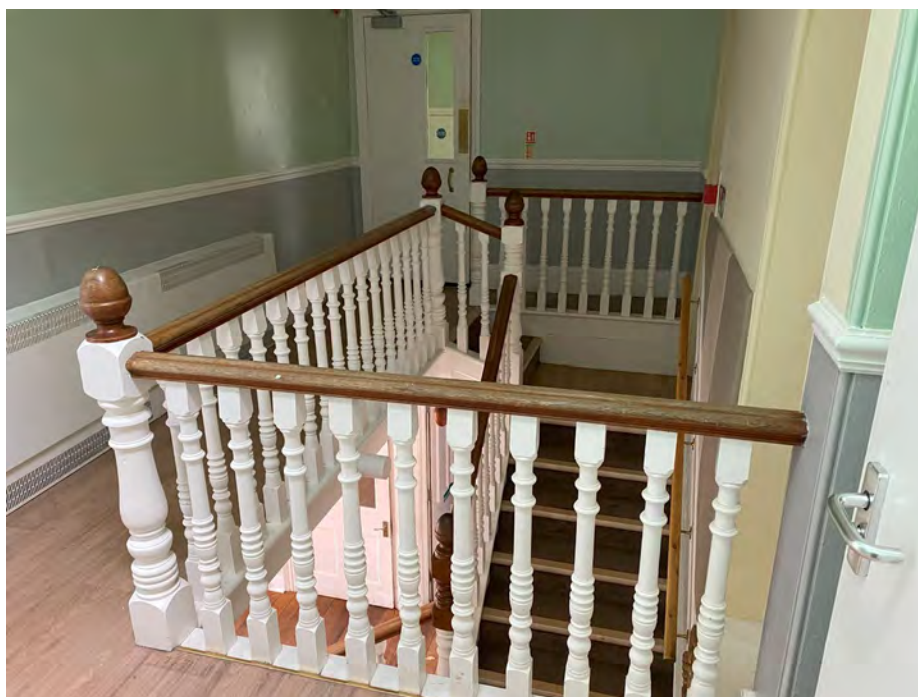
2.6: First floor landing with balustrade. New partition proposed to create entrance to unit 2 behind the existing balustrade. Door to right removed and opening blocked
