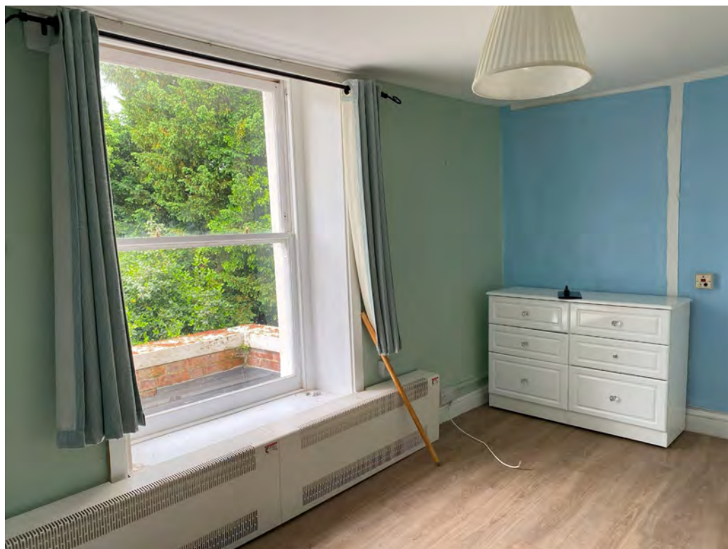
2.9: Typical second floor room with modern heating and windows and some evidence of timber framing
