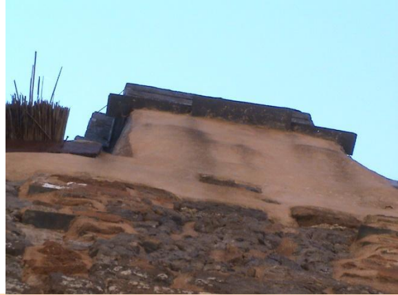
6. Gaps around chimney
