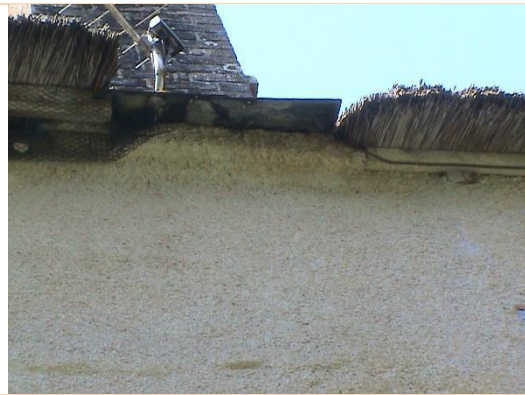
8. Crevices around and under slate
