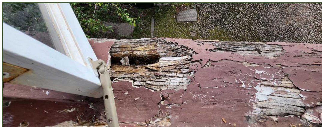
Figure 15. Bedroom 2 exterior sill demonstrating overall condition of sills throughout
