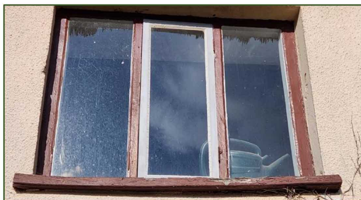
Figure 13. Bedroom 2 exterior, note warped/dropped sill
