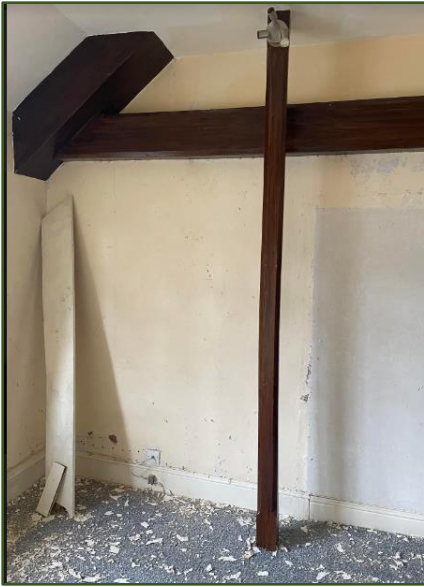
Figure 55. Bedroom 3 – upright support and false beam.
