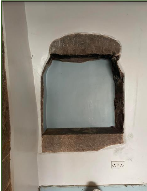
Figure 25. Blocked opening to rear of Abbotsford.
