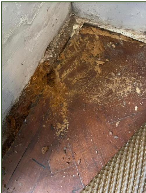
Figure 28. Sitting room rotted parquet flooring.
