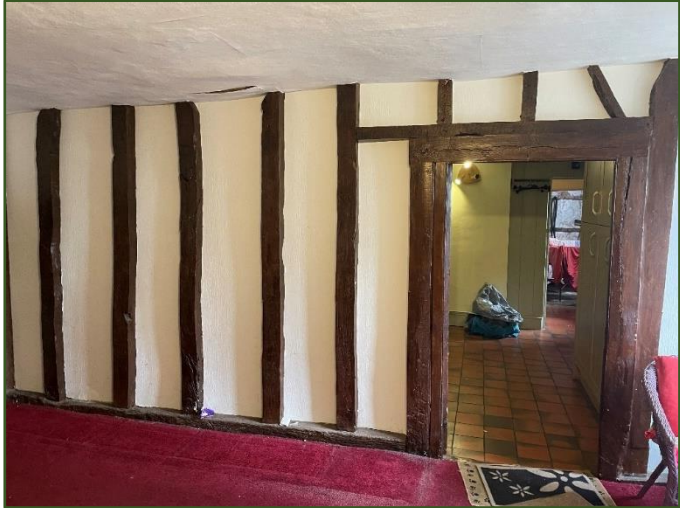
Figure 31. Dining room doorway (note frame timbers) leading to kitchen. Later installation of southern kitchen wall visible.
