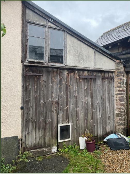
Figure 19. Workshop doors and window.
