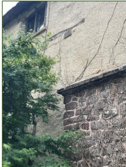
Figure 15. Rear elevation showing stonework, sitting room beam end and indentations in render.
