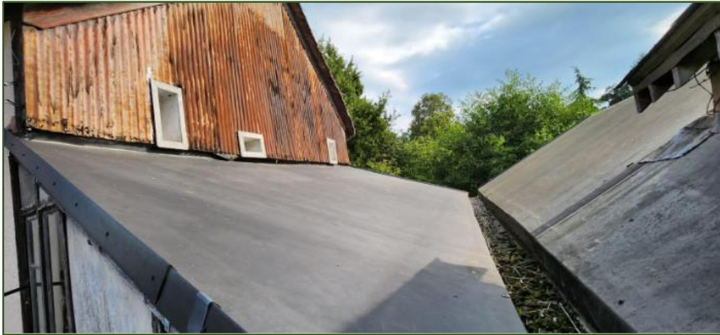
Figure 18. Valley roof, with left gable concealed under corrugated sheeting. Note 3 small window openings.
