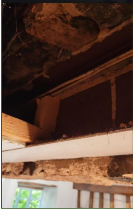
Figure 24. Large steel RSJ set behind existing stone lintel (fireplace). Note keystone to top of photo.
