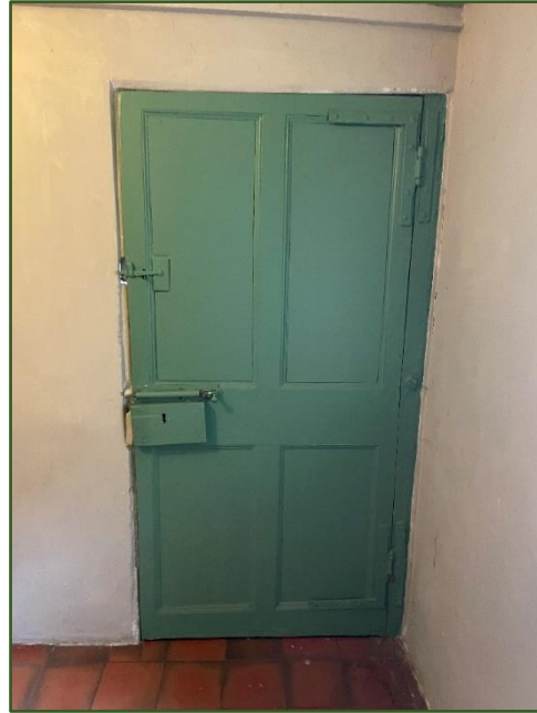
Figure 42. Timber 4-panelled door to workshop/store with iron hinges, latch and locking mechanism.
