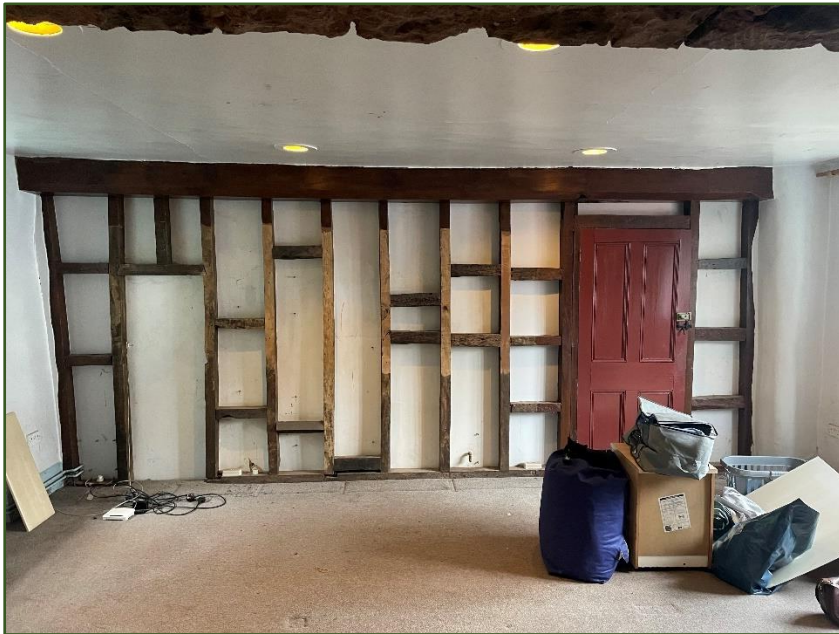
Figure 26. Wooden timber framed dividing wall with panelled door with modern Yale lock.
