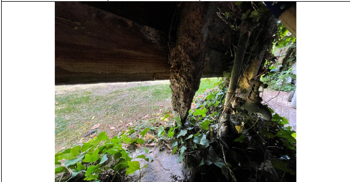
Photograph 14 Post Decay North Elevation
